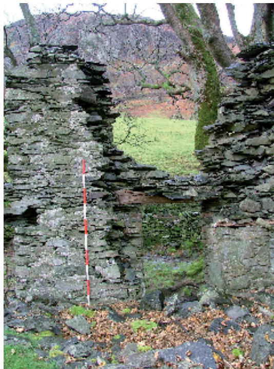
Plate 12 – View looking west from house interior showing surviving lintels of doorway and window, west wall, north end of house (Scale = 2m)
