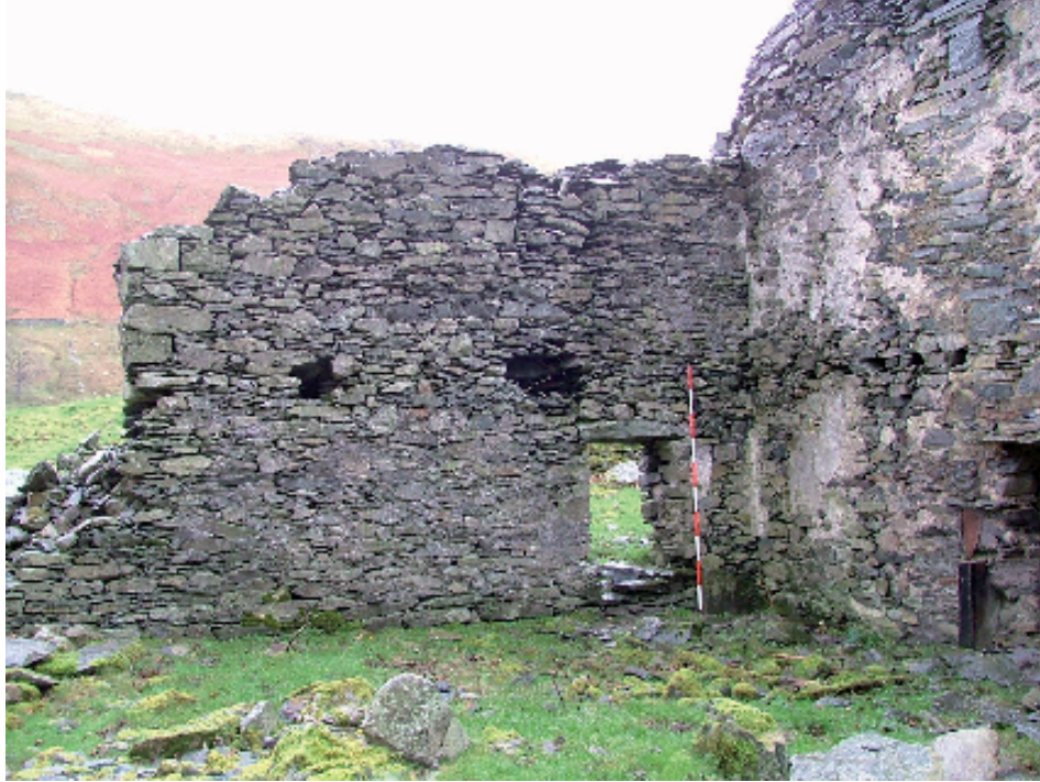
Plate 7 – View looking east of surviving section of house wall with window/low door, blocked first floor window and two large holes for former beams (Scale = 2m)
