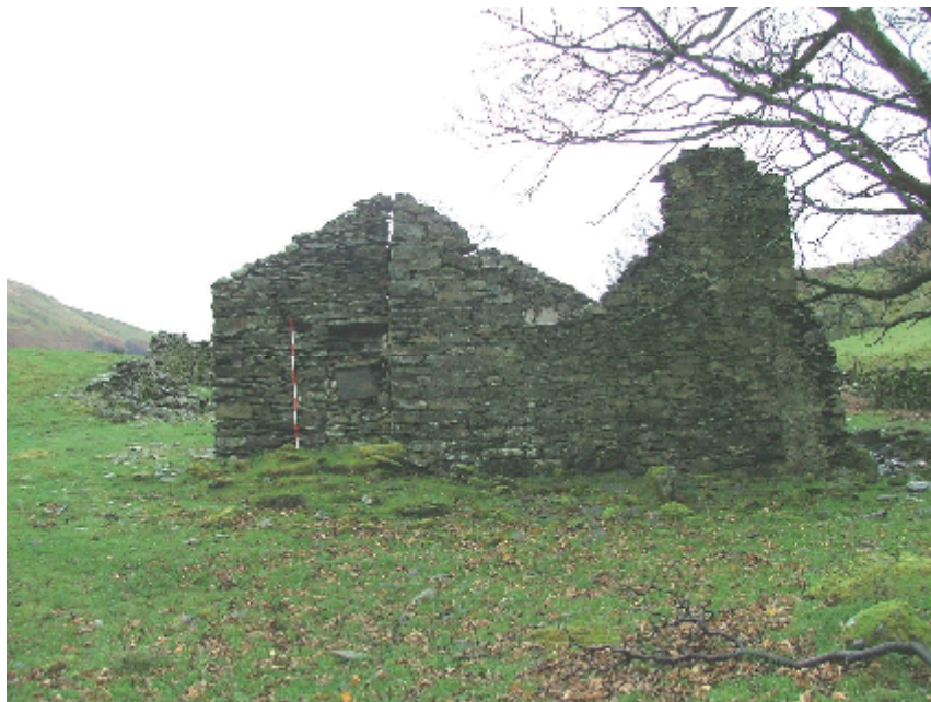
Plate 14 – View looking south of north end of house showing vertical line between main building and extension to the east, as well as the remains of a further extension against the north wall (possible privy/store/pig sty) (Scale = 2m)
