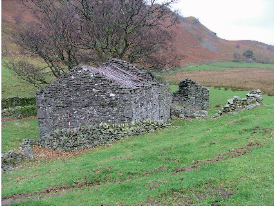
Plate 5 – View looking north showing the intact byre/stable at south end of Hen Howe
