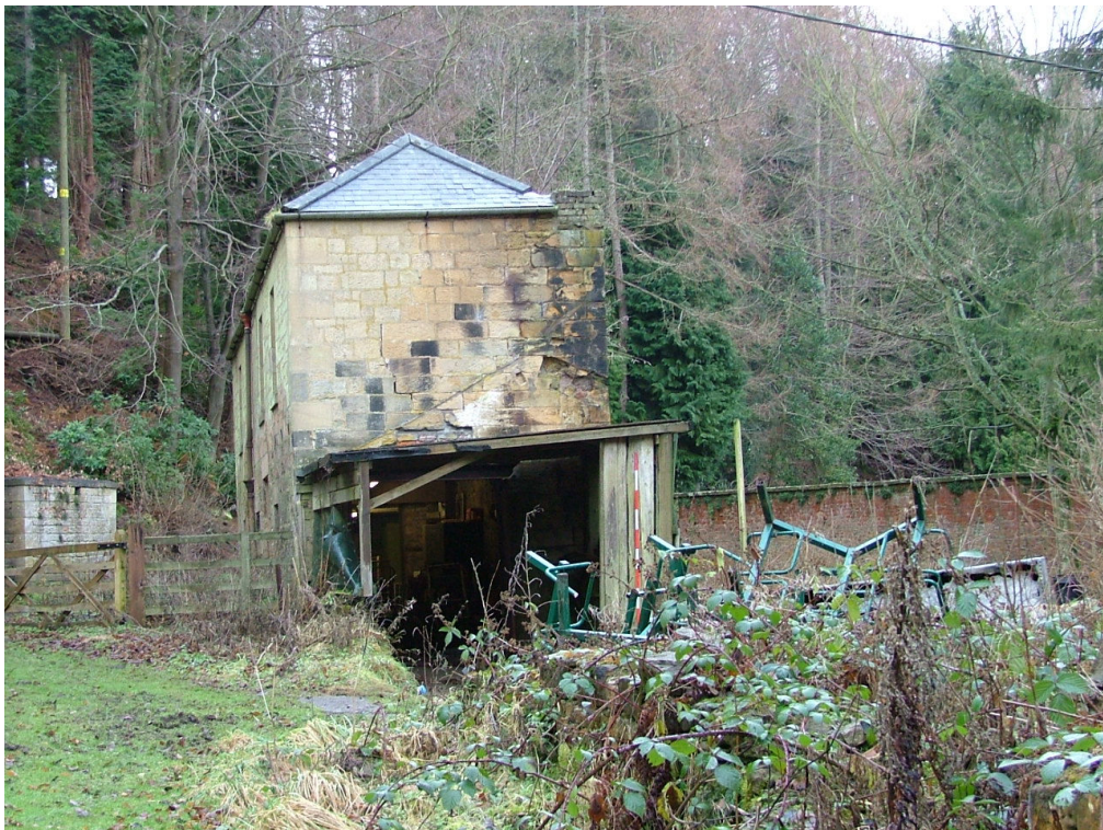
Plate 13 – West elevation of The Bothy showing the timber shelter and scarring of roof for a former single-storey building (Scale = 2m)
