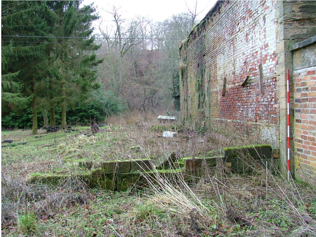
Plate 22 – View looking west showing the surviving masonry to the south side of The Bothy (Scale = 2m)
