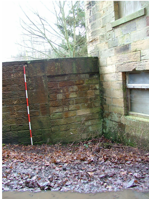
Plate 6 – Blocked doorway in garden wall, which terminates against the east elevation of The Bothy (Scale = 2m)
