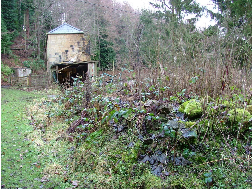
Plate 16 – View looking east towards The Bothy showing area of rubble and undergrowth providing evidence of a former building
