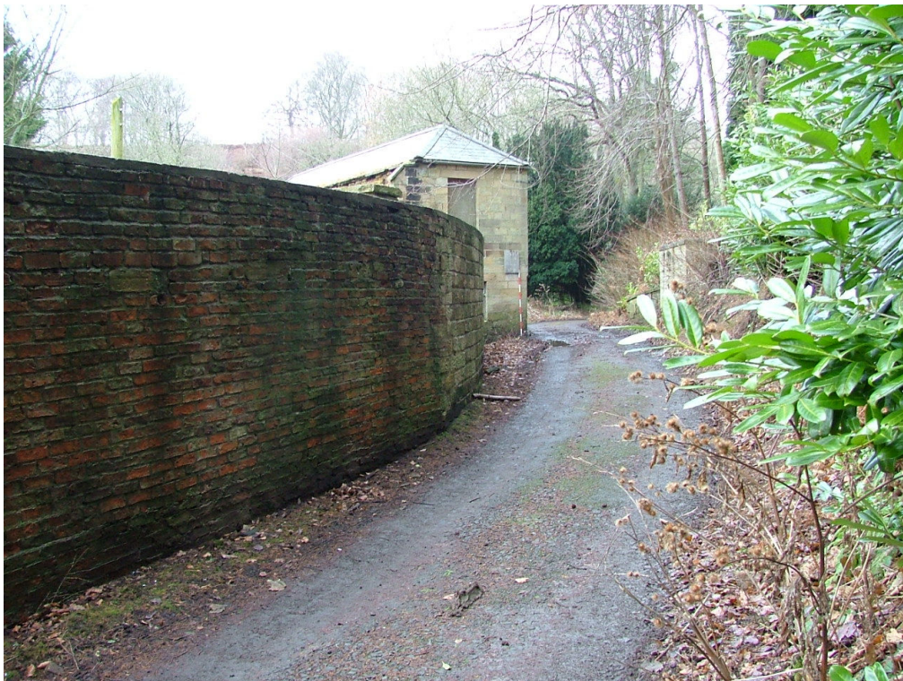
Plate 3 – View looking north-west showing the brick wall of the walled garden and track. The brick wall terminates against the east elevation of The Bothy
