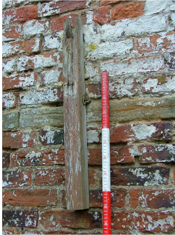
Plate 20 – Detail of one of the lengths of timber fixed to the wall with an iron fitting, south elevation of The Bothy
