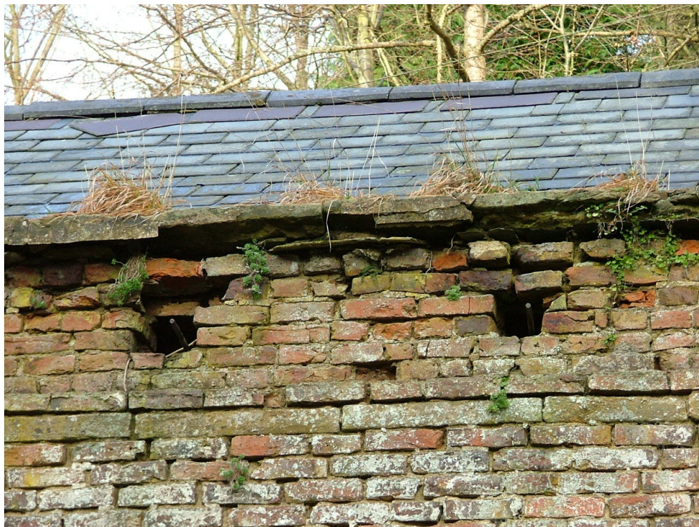
Plate 21 – Detail of holes at top of south elevation which may relate to the pitched roof of a glasshouse
