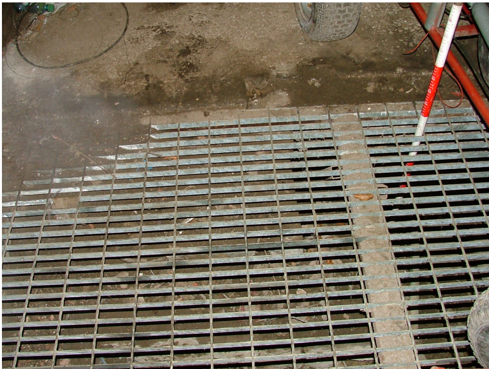
Plate 25 – Detail of lower ground level beneath modern grille, west end of The Bothy
