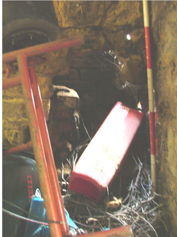
Plate 26 – Hole in south internal wall, possible location of a former fire or heater as shown by blackened masonry and brickwork
