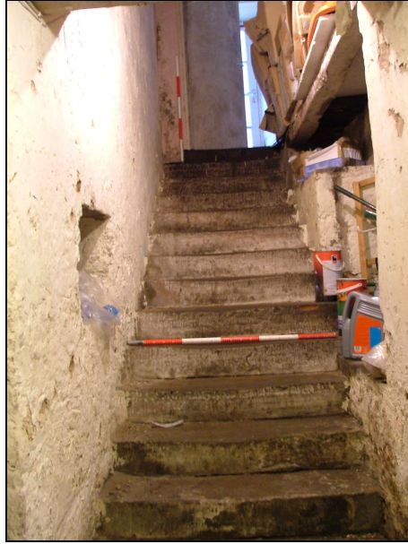
Plate 80 – View looking up the stone stairs from cellar to ground floor (Scales = 1m each)
