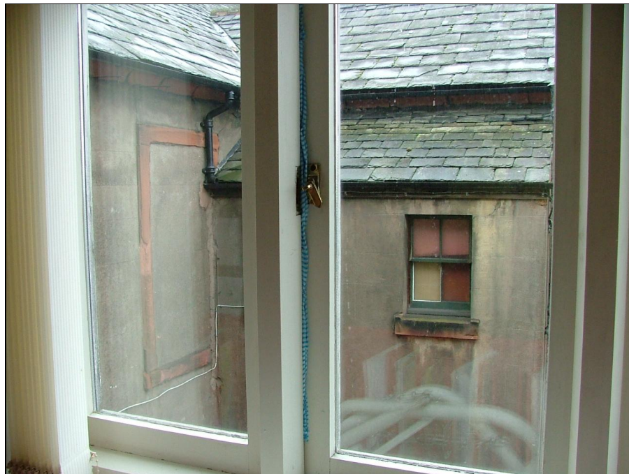
Plate 46 – View from pele tower of first floor extension over male toilets which partly obscures the right-hand jamb of window on the north-west elevation of mansion house
