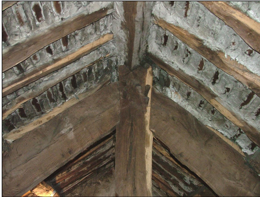
Plate 75 – Detail of one of the king-posts showing wooden pegs and v-shaped notch in top of king-post to hold the ridge beam, attic of mansion house
