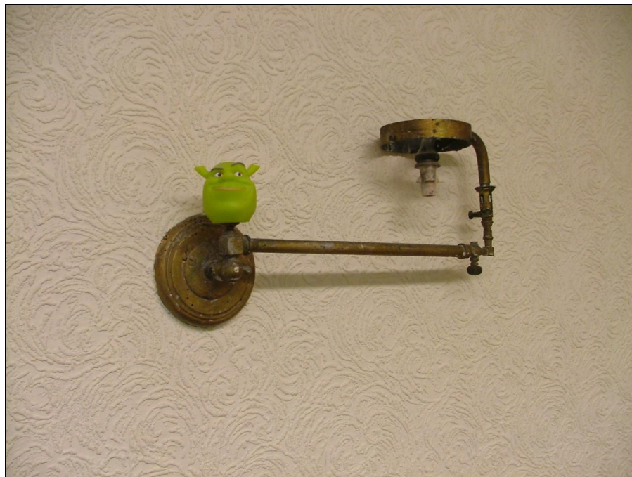
Plate 19 – Remains of a gas light complete with 'Shrek', first floor of pele tower
