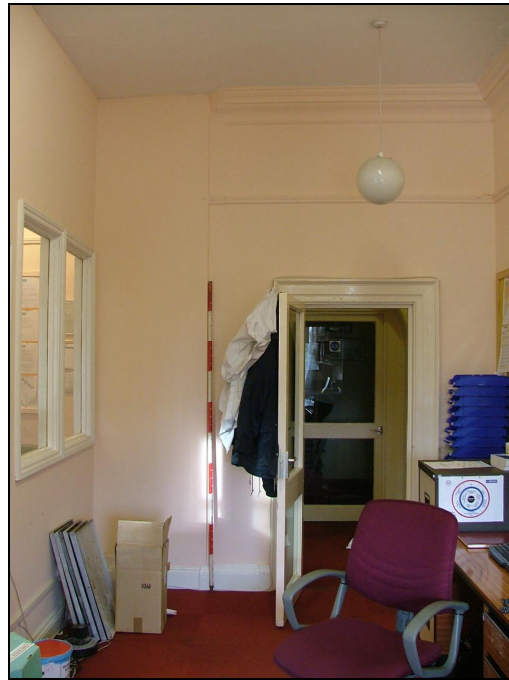
Plate 64 – First floor of mansion house showing termination of coving and picture rail (Scale = 2m)
