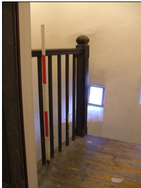
Plate 22 – Newel post, handrail and balusters, top of spiral staircase in pele tower (Scale = 1m)
