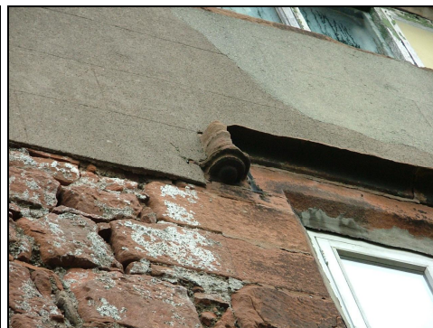
Plate 11 – Second floor label stop
