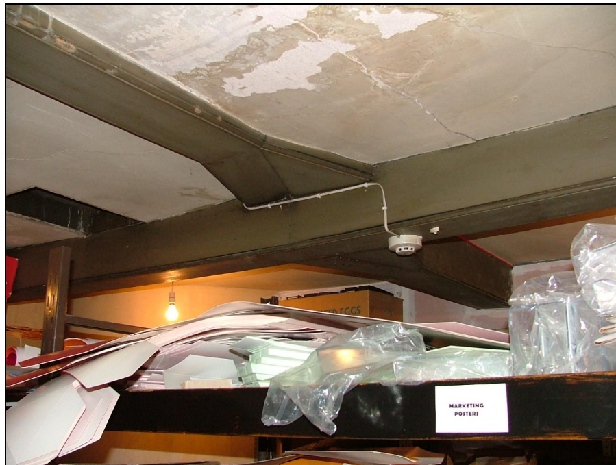
Plate 24 – Third floor of pele tower, beams in ceiling supporting central post of pyramidal roof
