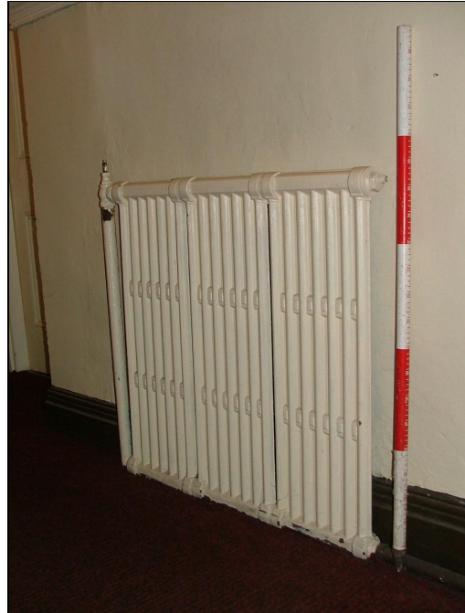
Plate 53 – Detail of radiator, ground floor corridor of mansion house (Scale = 1m)
