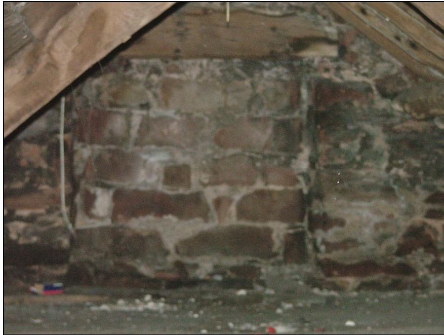
Plate 73 – View of the blocked attic window with timber lintel in stair tower
