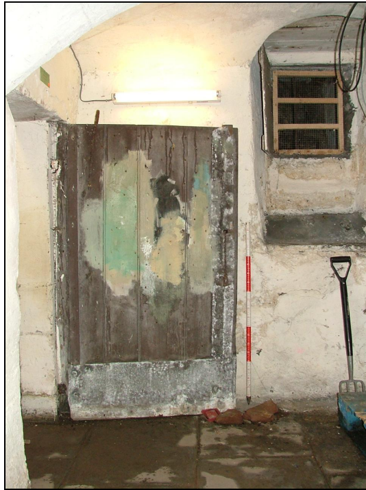
Plate 90 – Door to northern cellar room showing repair work using metal sheets (Scale = 1m)
