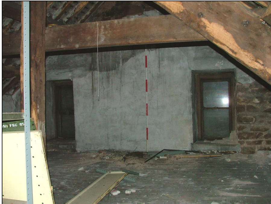
Plate 79 – South-west wall of attic showing two, 2-pane sash windows (now blocked externally)
