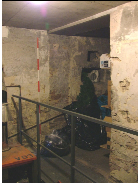
Plate 16 – Ground floor of pele tower showing scarring of former masonry cross wall with niches set in wall to the right (Scale = 2m)
