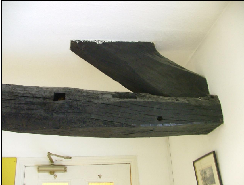
Plate 35 – Part of roof truss made from reused timber, first floor of cottage
