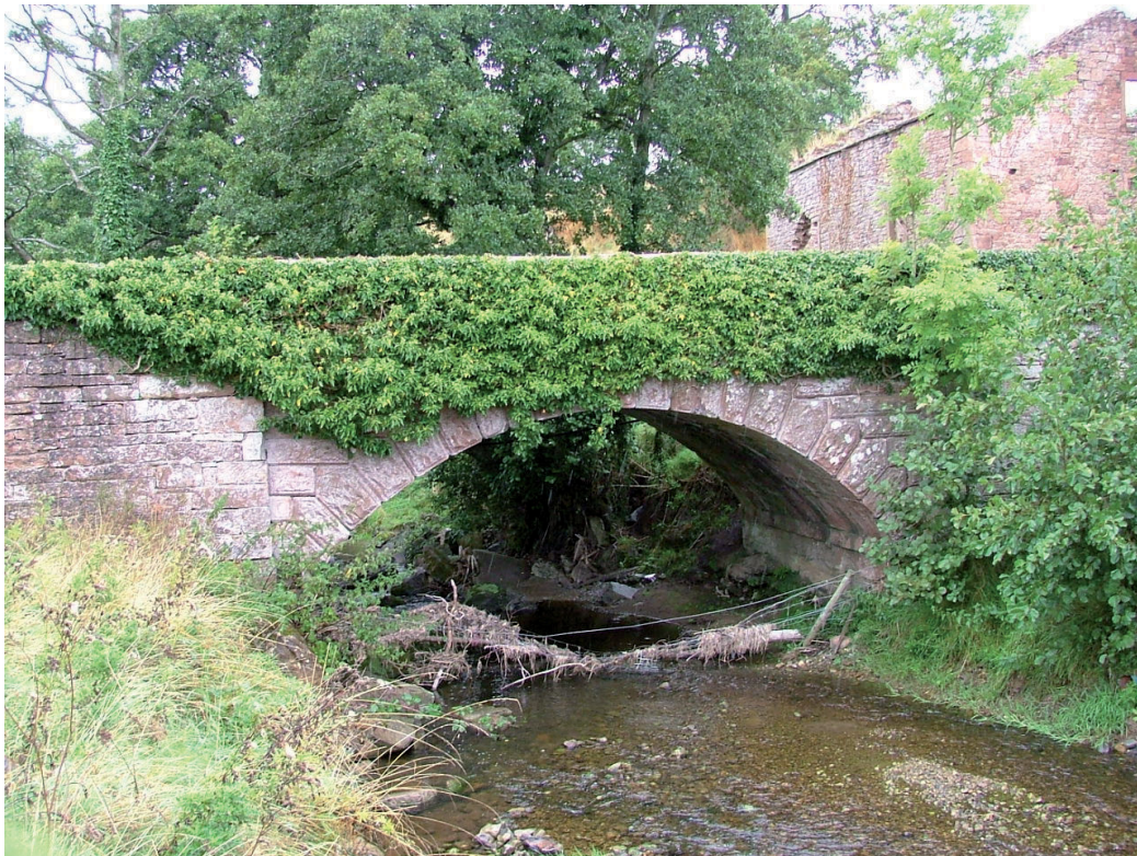
Plate 66 – The Mill Bridge looking north, with the mill to the right of photograph
