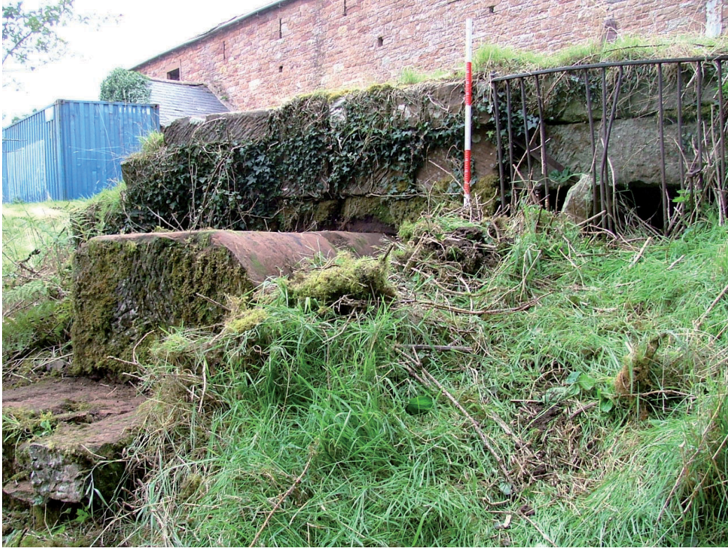
Plate 35 – Culvert with iron grill (to the right of ranging pole) and remains of the weir for the sheep dip
