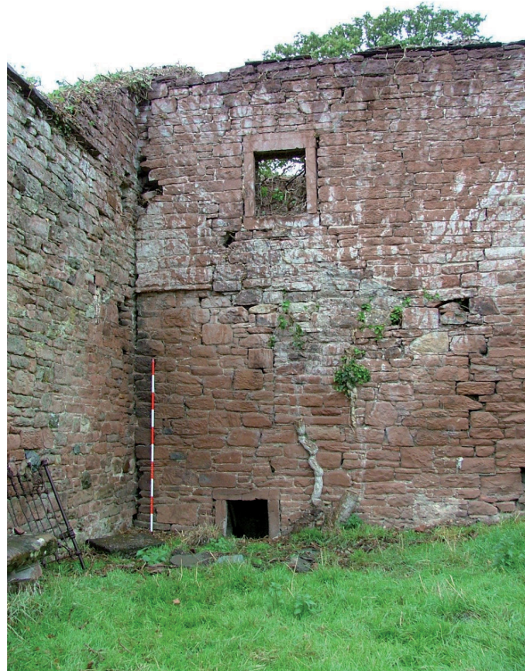
Plate 51 – Western end of south facing elevation of rear wing showing window to corn dryer, blocked and upper windows and difference in stonework
