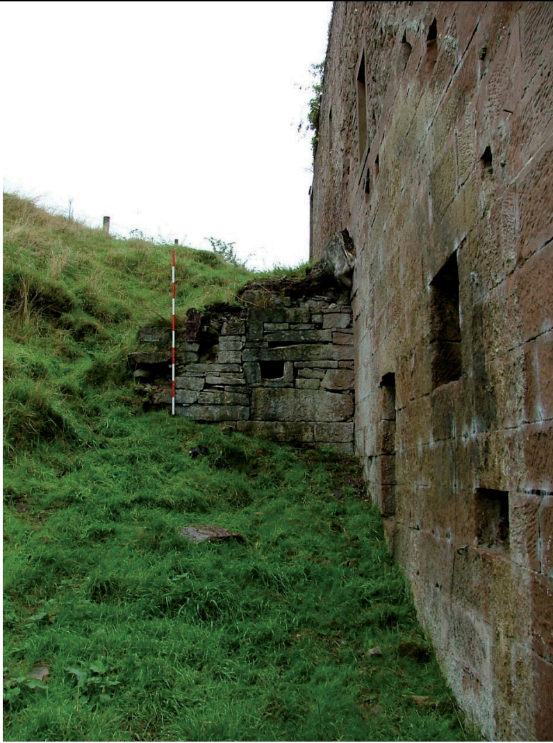
Plate 46 – The remains of the Head Race complete with an exit hole for water
