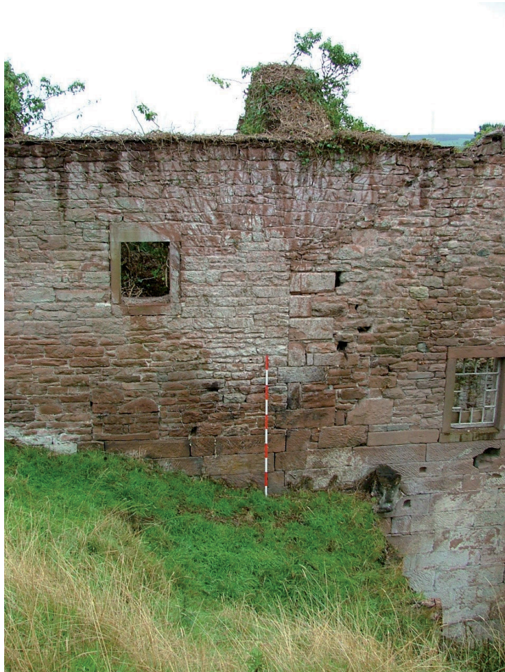
Plate 47 – Northern elevation of mill showing construction break between the main mill and the addition
