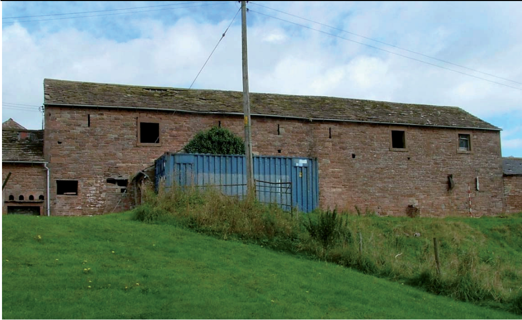
Plate 4 – South facing elevation of the large barn ‘A’ showing roof of sandstone tiles
