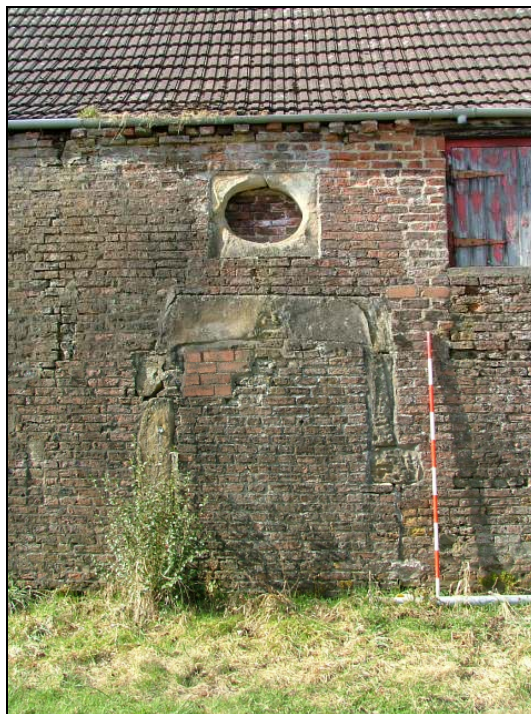
Plate 12 – Blocked doorway with dressed stone surround and œil-de-boeuf window above (Scale = 2m)
