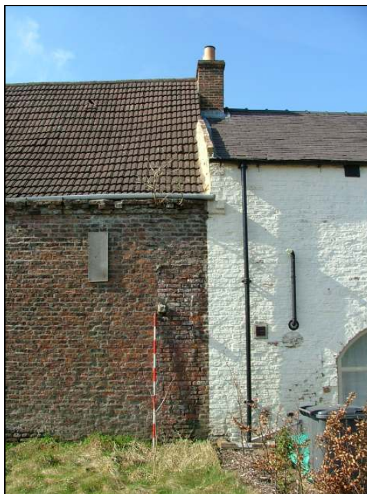
Plate 16 – North end of east elevation showing some evidence for a possible buttress formerly located against this wall (Scale = 2m)
