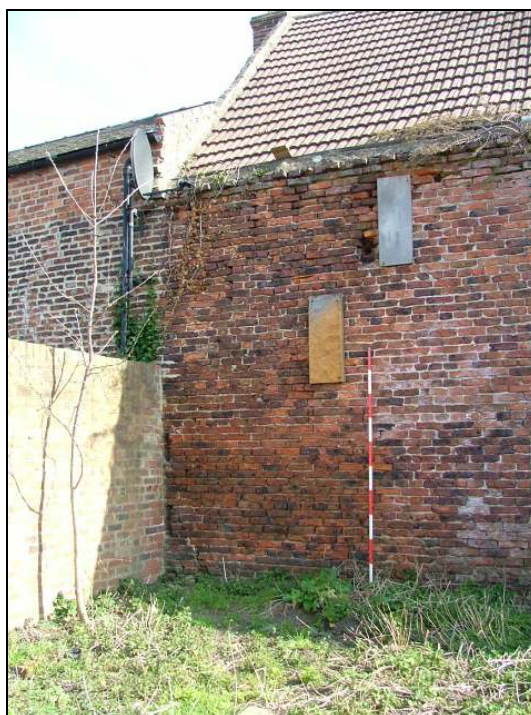
Plate 25 – North end of west elevation showing boarded ventilation slits and continuation of brickwork into Farm Cottage. Note the heightening of the wall of Farm Cottage which creates a different pitch roof (Scale = 2m)
