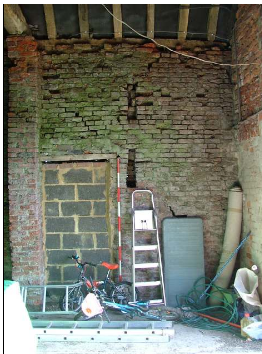
Plate 33 – Blocked doorway and ventilation slits, south end of east internal elevation (Scale = 2m)
