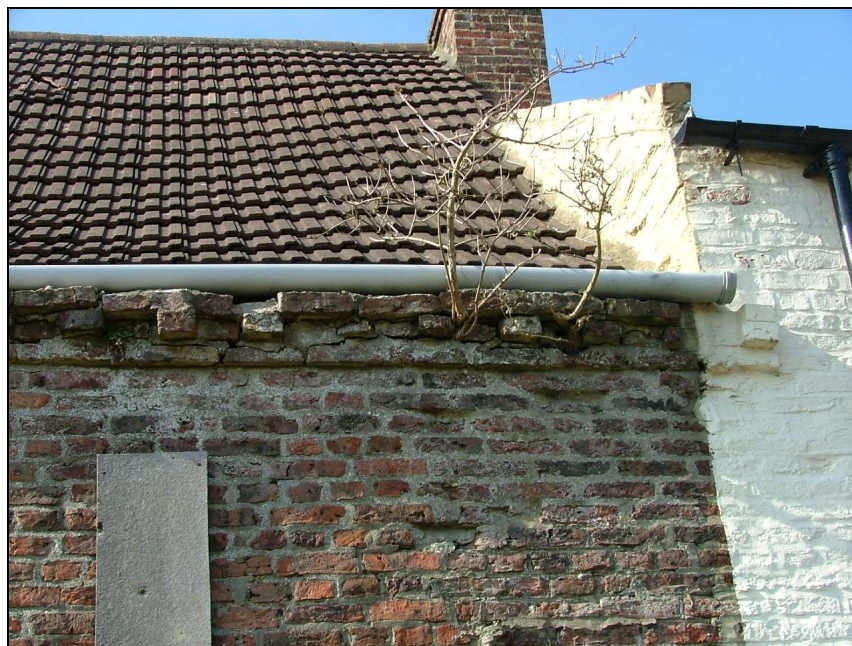
Plate 9 – Detail of the dentilated brickwork at eaves level, note that it extends to the property next door indicating that Farm Cottage (or at least part of it) was once a continuation of the barn
