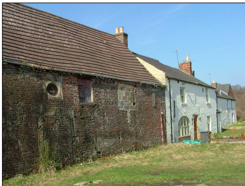
Plate 7 – View looking north-west of the east elevation of the barn, with Farm Cottage to right of photograph (Scale = 2m)
