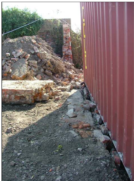
Plate 41 – View looking south of demolished brick wall to south of barn (Scale = 2m)
