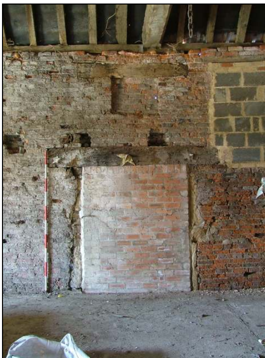
Plate 36 – Blocked doorway with possible holes for floor beams above, west elevation (Scale = 2m)
