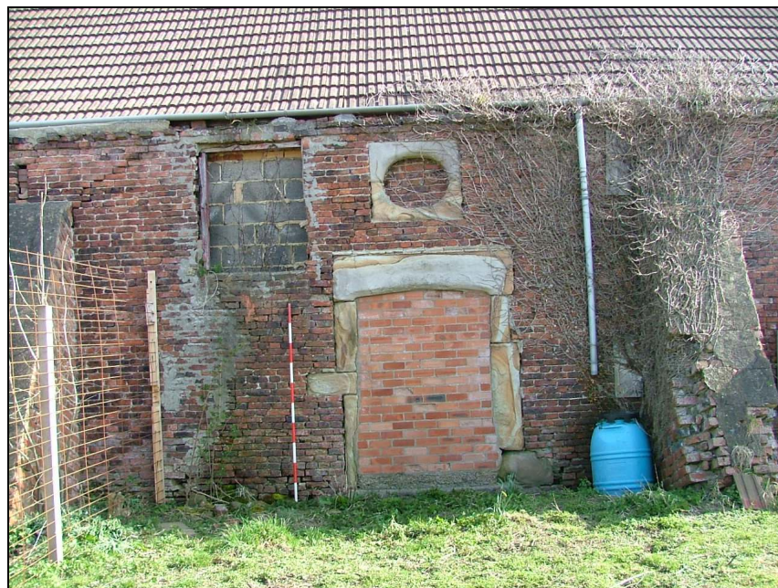
Plate 21 – Doorway and œil-de-boeuf, with later pitching window to left, west elevation (Scale = 2m)
