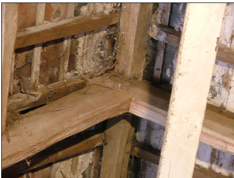
Plate 12 – Detail of wooden pegs at apex of one of the roof trusses, West Barn
