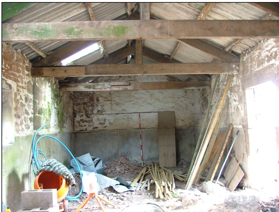
Plate 46 – View looking east of the interior of the South Range (byre) (Scale = 2m)
