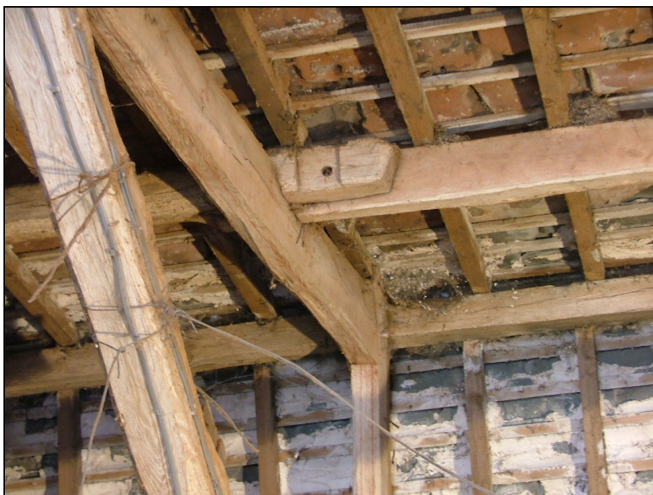
Plate 11 – Detail of one of the purlin ends showing evidence of re-use, West Barn
