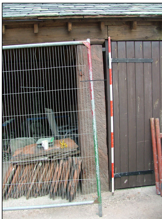
Plate 35 – External view of one of the sandstone columns, south elevation of North Range (Scale = 2m)
