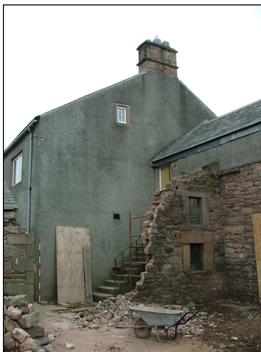
Plate 55 – North gable of main house showing stone stairs and remains of extension with windows (Scale = 2m)
