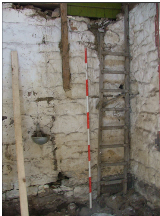
Plate 30 – Wooden ladder against masonry wall which divides the ground floor of the East Byre, formerly provided access to the hayloft above (Scale = 2m)
