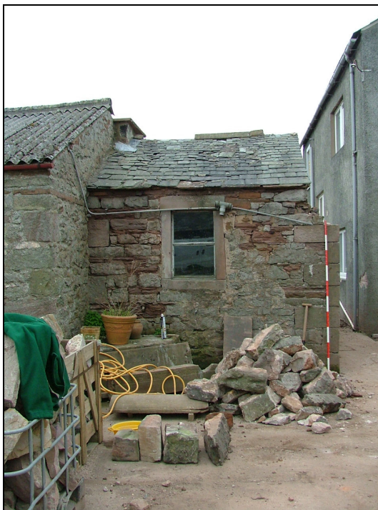
Plate 50 – North elevation of wash-house with a possible plinth for milk churns to the left of photograph (Scale = 2m)
