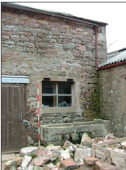
Plate 23 – One of the windows in the west elevation of the East Byre (Scale = 2m)
