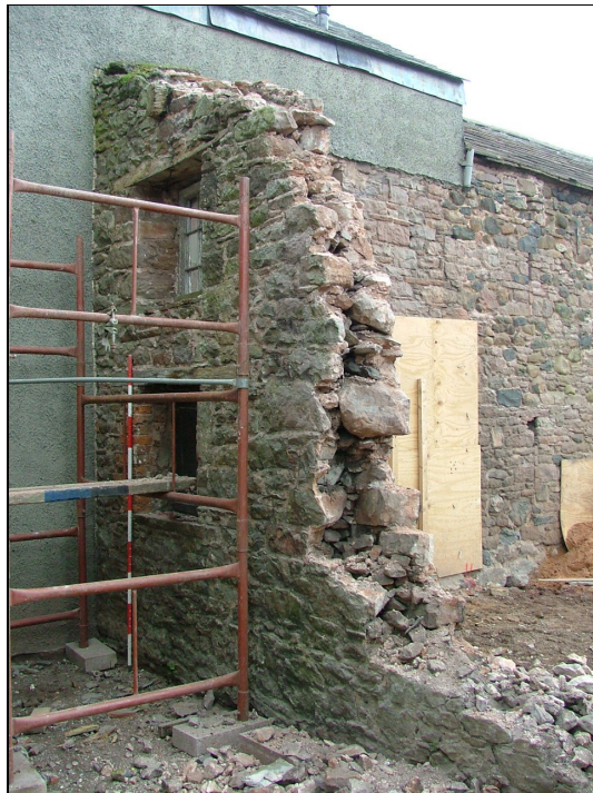
Plate 58 – View looking north-west of the remaining section of wall of the outshut showing the render on the back wall and above the location of a former lean-to (Scale = 2m)
