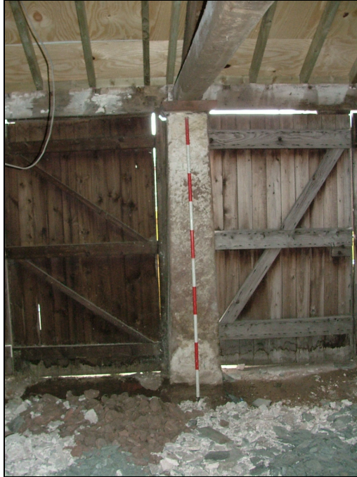
Plate 36 – Internal view of one of the sandstone columns, south side of North Range (Scale = 2m)
