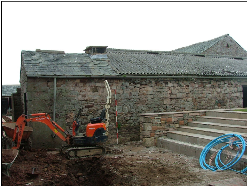
Plate 48 – West end of South Range (south elevation) showing slate roof over wash-house and remains of chimney stack (Scale = 2m)
