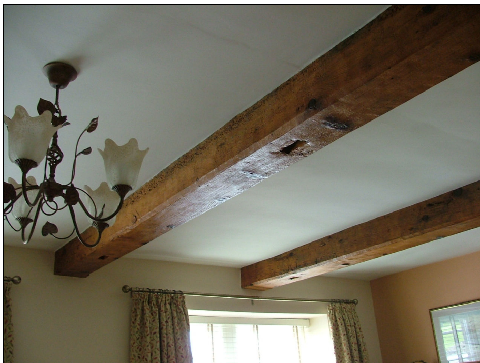
Plate 60 – Beams in ceiling of lounge showing redundant mortice holes for possible stall divisions
