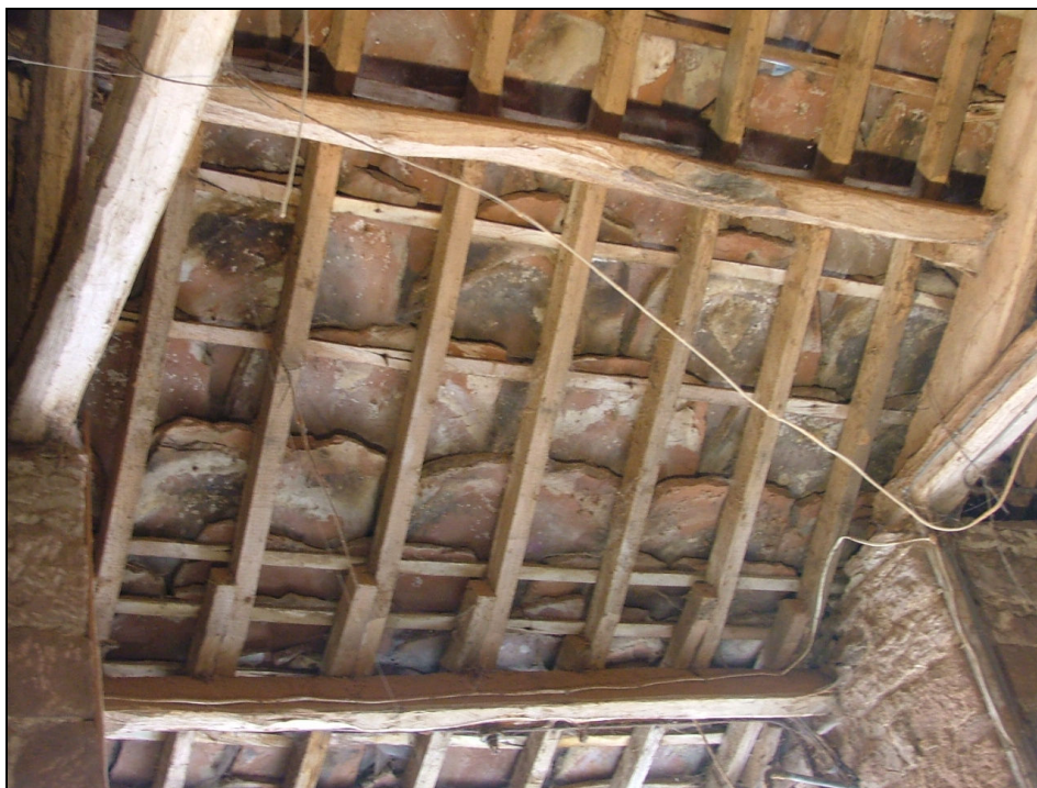
Plate 13 – Detail of east side of West Barn roof showing rounded tops of sandstone tiles and redundant peg holes
