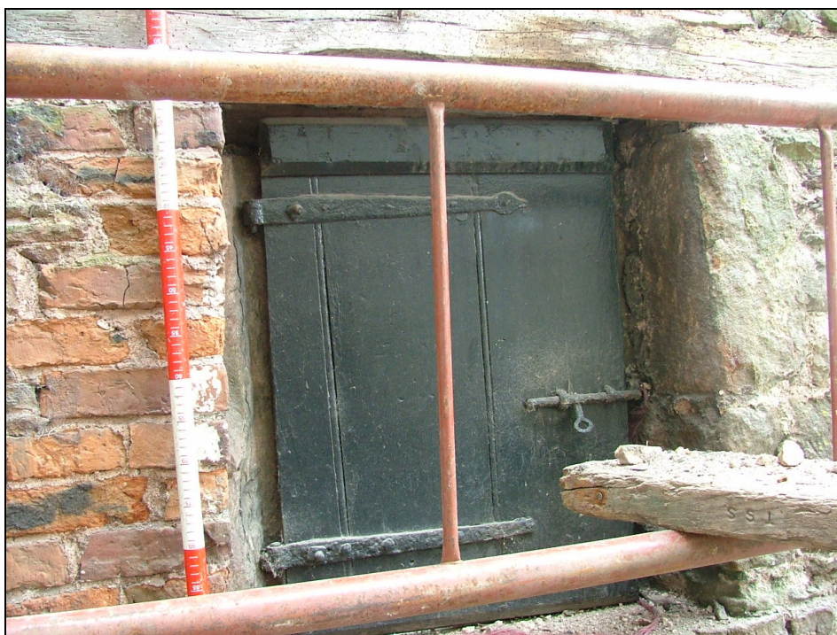
Plate 59 – Detail of the wooden door of the ground floor window to outshut
