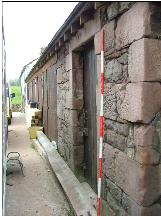
Plate 37 – View looking west along the south elevation of the North Range showing one of the door surrounds to a stable/loose box
