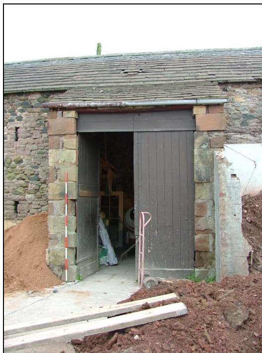
Plate 8 – Large double doorway set in a projecting porch, east elevation of West Barn (Scale = 2m)
