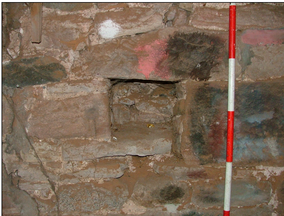
Plate 17 – Niche in projecting porch way, West Barn (Scale is in 20cm graduations)
