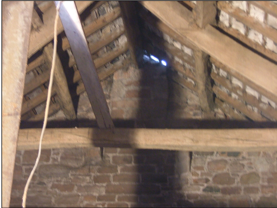
Plate 19 – Projecting masonry at apex of south internal gable of West Barn indicative of chimney stack located in the building to the south
