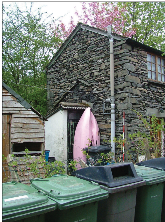
Plate 34 – West elevation of small cottage showing line of a former roof (Scale = 2m)
