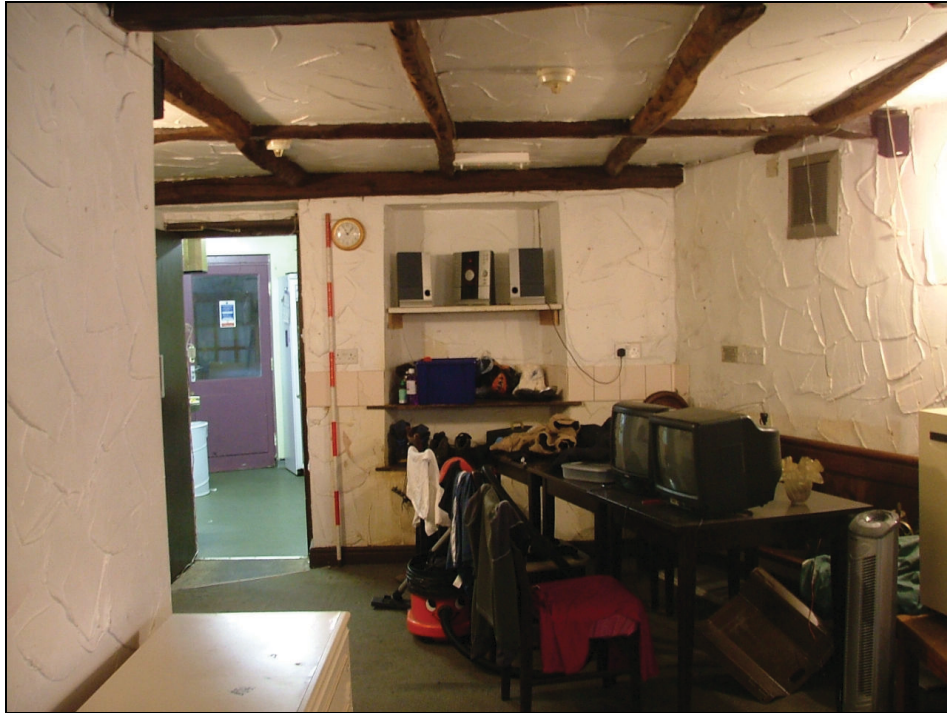
Plate 26 – View looking west of the ground floor of Mill Cottage showing a blocked window (Scale = 2m)
