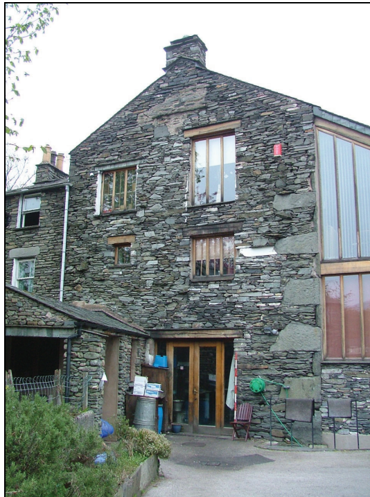
Plate 24 – West elevation of the Glass House Restaurant with the two windows left of the drainpipe located in the west elevation of Mill Cottage (Scale = 2m)
