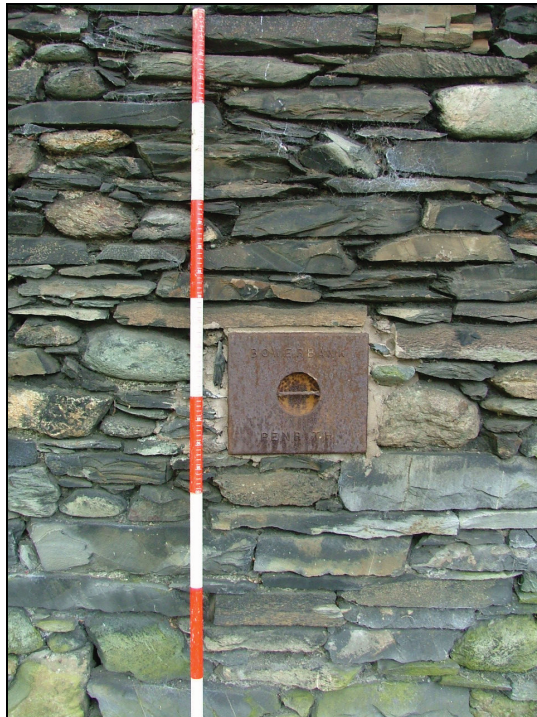
Plate 37 –presumably used to access the flue of a fireplace (Scale is in 20 cm graduations)
