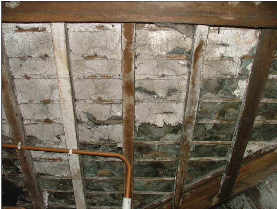
Plate 32 – Underside of slate roof showing sections of ‘torching’ applied to reduce draughts
