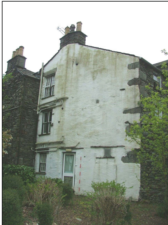
Plate 19 – Part of the north elevation showing the different phases of building (Scale = 2m)
