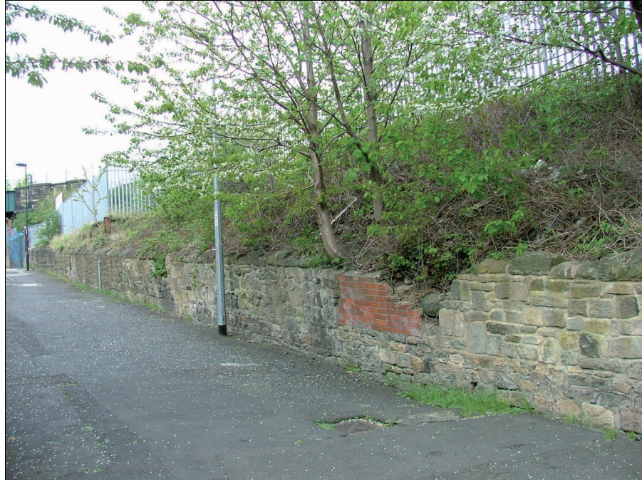
Plate 8 - View looking north along the boundary wall to the west of the site
