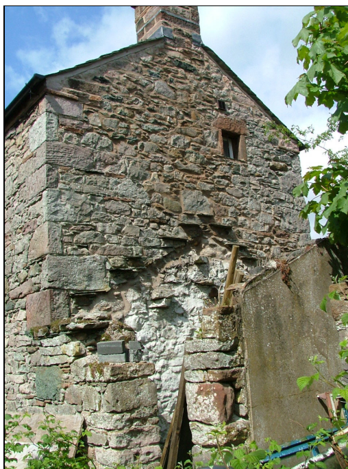
Plate 44 – East gable of two-storey building to the east of Midtown and the scarring of the roofline of the single-storey range
