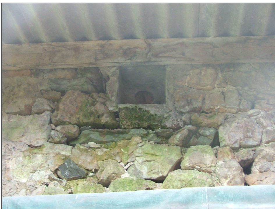
Plate 39 – Detail of one of the ventilation holes along the top of the south elevation, Building 3
