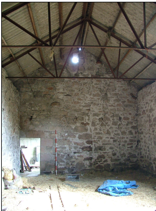
Plate 25 – View looking north of the interior of Building 2 showing a doorway to Building 3 and a vertical construction break in the north gable (Scale= 2m)
