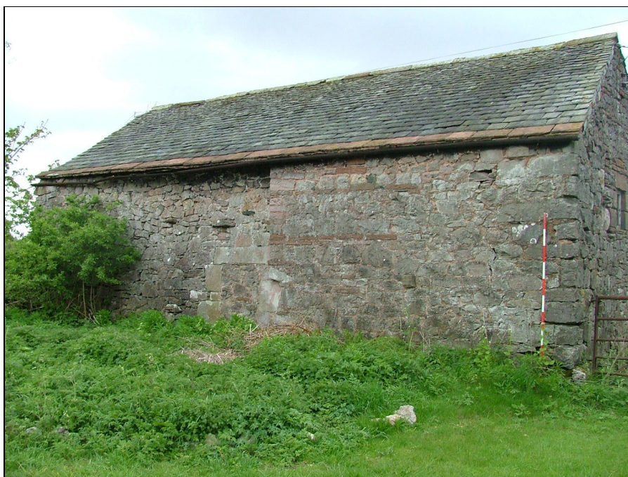
Plate 6 – North-west elevation of Building 1 showing blocked doorway and vertical construction break (Scale = 2m)
