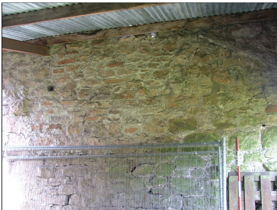
Plate 18 – Diagonal line of a former roof against the east elevation of Building 2
