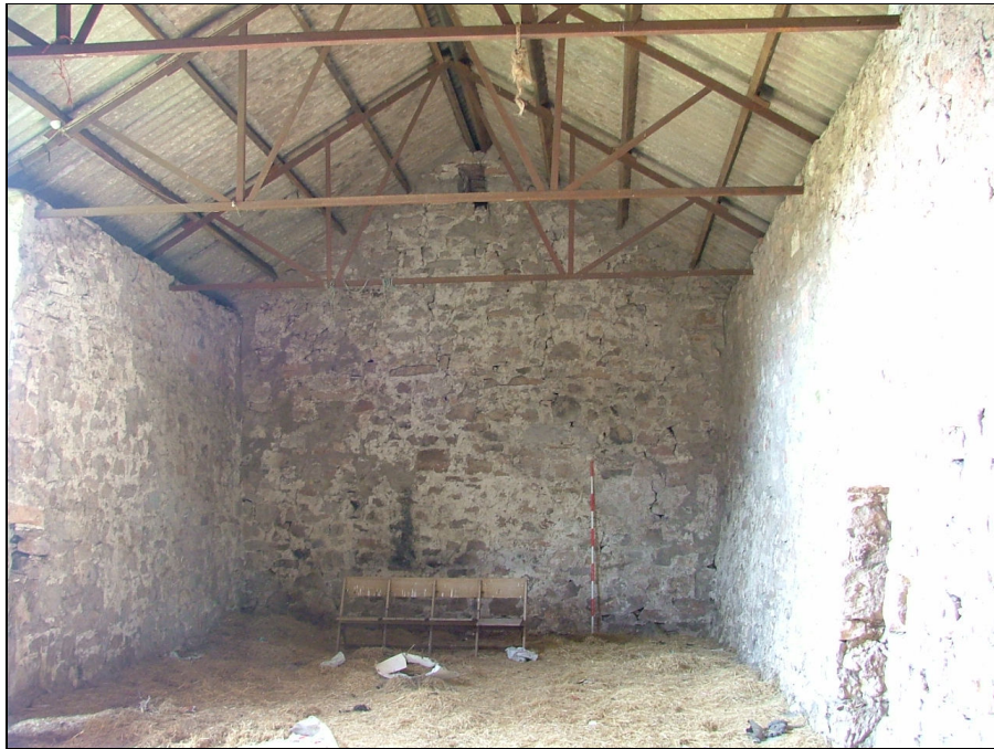
Plate 24 – View looking south of the interior of Building 2 showing the modern roof structure (Scale = 2m)
