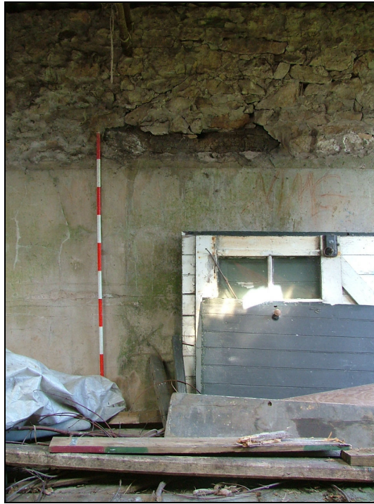
Plate 40 – Wooden lintel of the blocked doorway in the north elevation, Building 3 (Scale = 2m)
