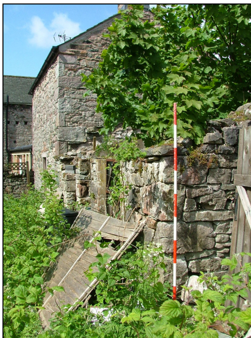
Plate 43 – View looking west showing a two-storey building, which may now form part of Midtown, and the remains of a single-storey range, all located to the north of Building 3 (Scale = 2m)
