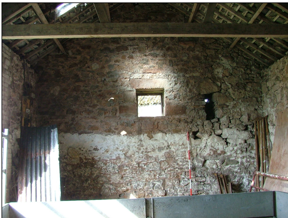
Plate 11 – South-west internal wall of Building 1 showing part limewashed walls and window (Scale = 2m)
