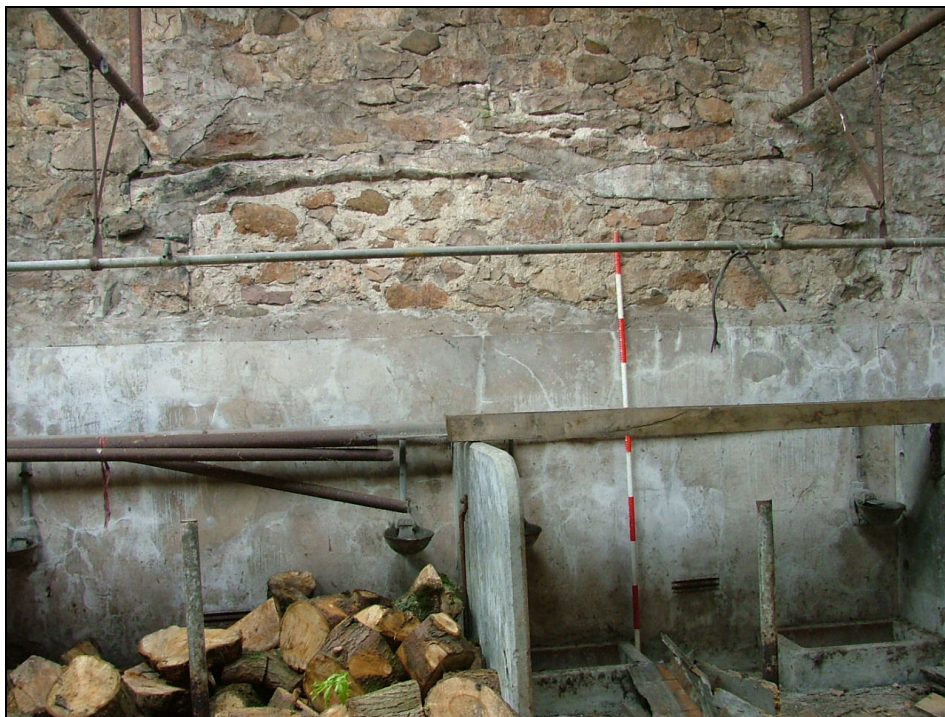
Plate 38 – South internal wall of Building 3 showing the lintels of a former doorway/window (Scale = 2m)
