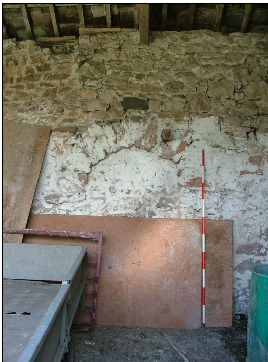
Plate 12 – Blocked doorway with arched head, north-west internal elevation of Building 1 (Scale = 2m)
