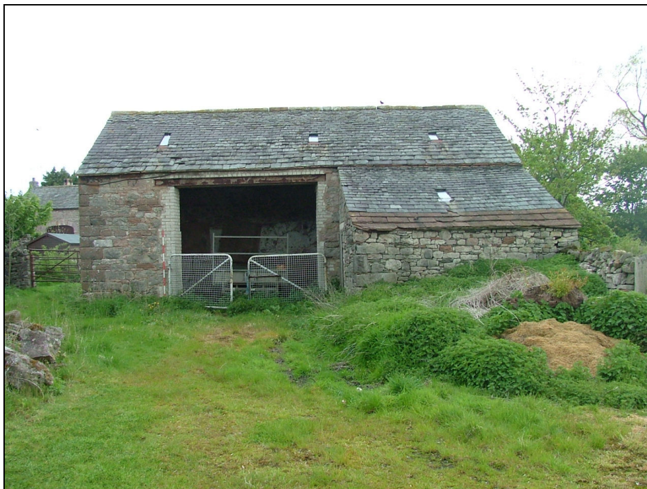
Plate 1 – South-east facing elevation of Building 1 showing the outshut to the eastern side
