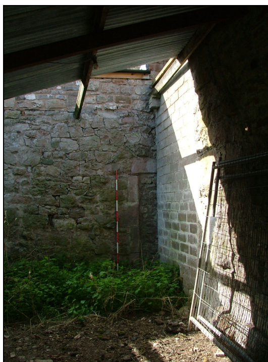
Plate 20 – Blocked doorway in the north wall of The Mains as seen from the east elevation of Building 2 (Scale = 2m)
