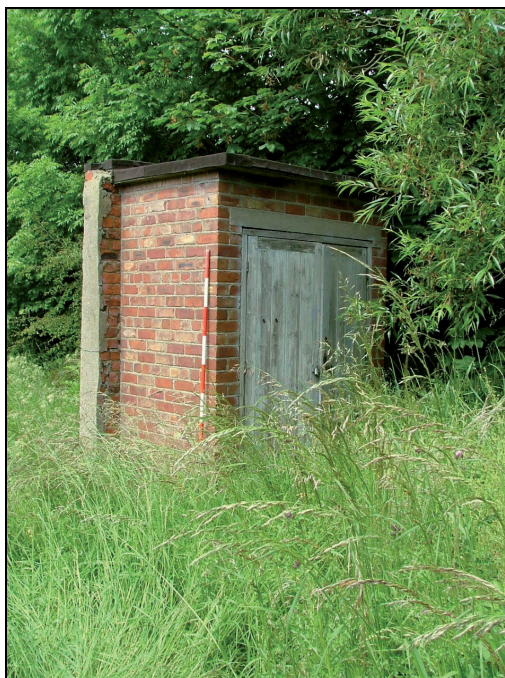
Plate 10: Brick-built structure on north side of western section of proposed development area, possible generator house? (Scale = 2m)
