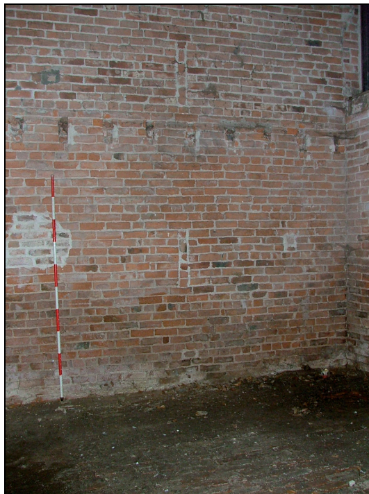
Plate 28: Joist holes and blocked ventilation slits in east wall of barn, Building 1 (Scale = 2m)
