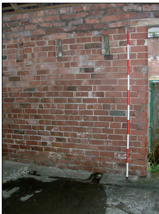
Plate 59: Interior of Building 4 showing concrete floor, ventilation slits and curved edge to the door jamb (Scale = 2m)
