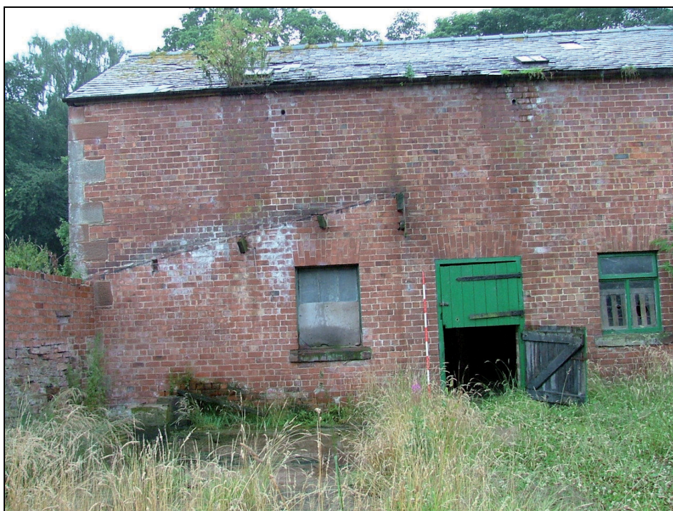
Plate 15: South end of east elevation of Building 2 showing scarring of a former roofline (Scale = 2m)
