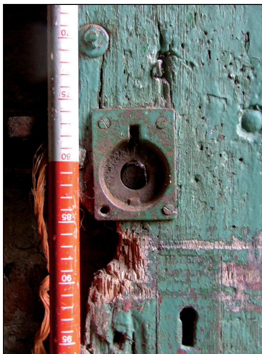
Plate 23: Detail of 'push button' door latch, large doorway to barn, Building 1 (Scale is in 1cm graduations)
