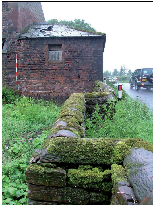
Plate 65: East elevation of Building 5 showing masonry plinth, quoins and window and boundary wall (Scale = 2m)
