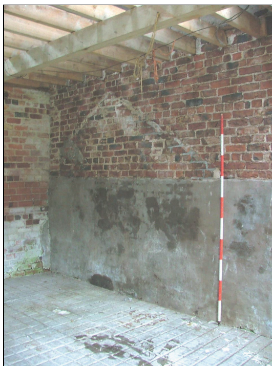
Plate 29: Scarring of a former single-storey building, north internal wall of Building 2 (Scale = 2m)
