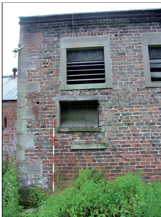
Plate 44: Window in south end of east elevation, Building 3, replaced an earlier window (Scale = 2m)
