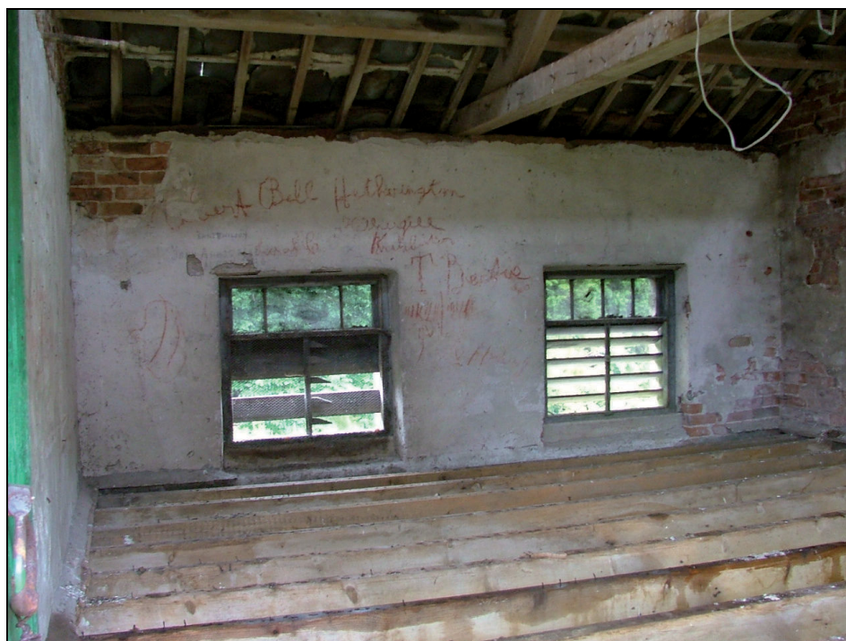
Plate 55: East wall of first floor granary, Building 3 showing louvered windows and graffiti
