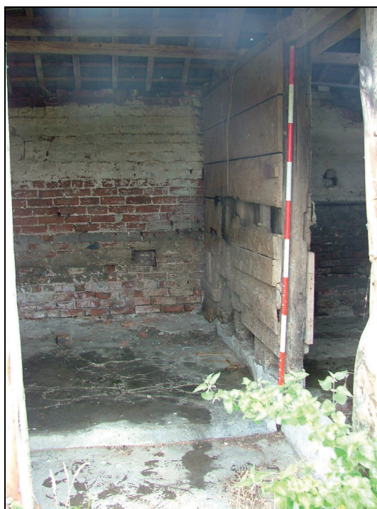
Plate 75: View of loose box, west end of Building 5, showing brick interior walls (Scale = 2m)
