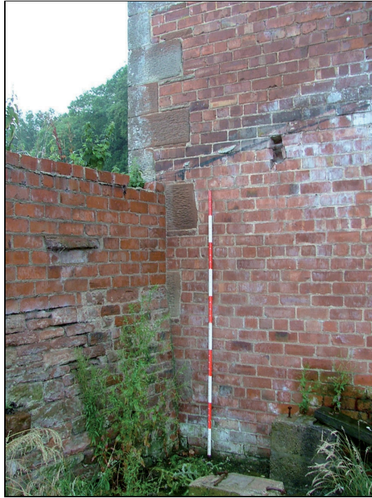
Plate 16: South end of the east elevation of Building 2 showing brick wall of a former building against the quoins of Building 2 (Scale = 2m)
