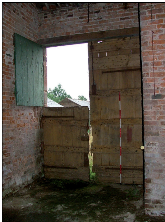
Plate 20: Internal view of doorway into barn, east elevation of Building 1 (Scale = 2m)
