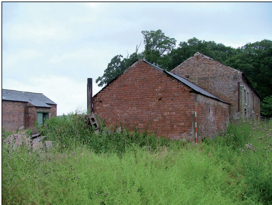
Plate 42: View looking north showing the south gables of Building 4 (in the foreground) and Building 3 (Scale = 2m)
