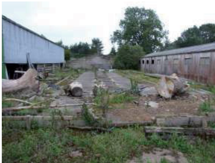
Plate 6: Two of the standing buildings present on site with a demolished building in the middle. The building on the right is shown in Plates 2 and 4, looking east, southeast
