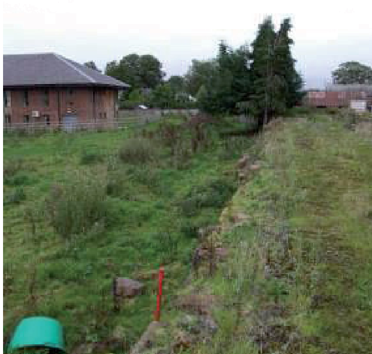
Plate 5: Boundary wall to the built up area, looking northeast. Note the rocks on the ground appeared to be tumble from the wall, the aforementioned surgery is to the left-hand side of the photo
