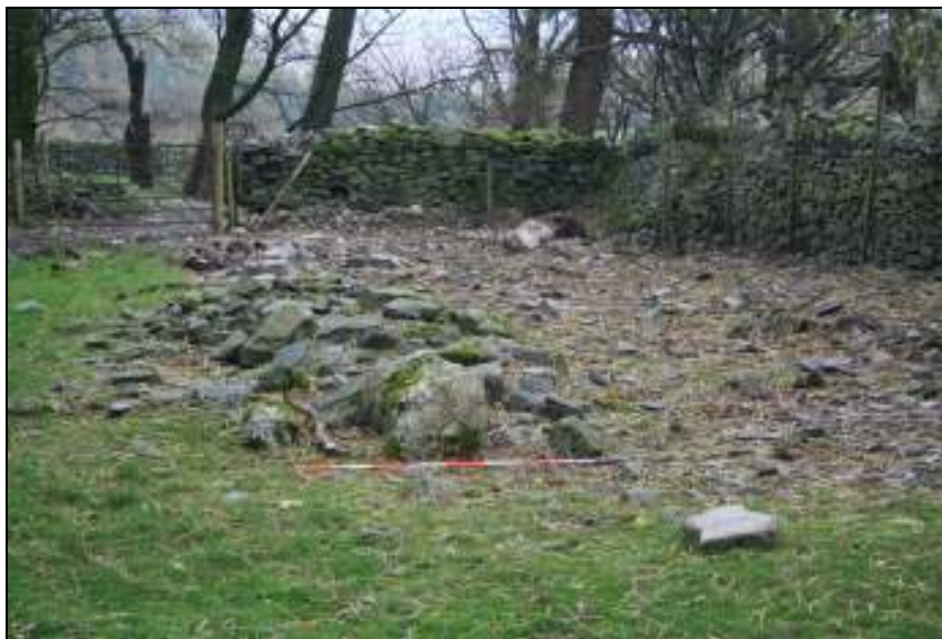
Plate 5: Foundation wall of a rectangular building on the north side of the site, the subject of the trial trench evaluation (looking west)
