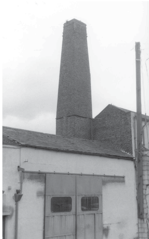
Plate 4: Chimney stack adjacent to office units. The chimney is probably the remains of the tallest of two stacks shown in a drawing of 1900 and surviving in a photograph of c. 1907.
