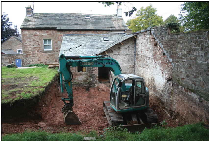
Plate 6: Excavation of the artificially-lowered area on the east side of the development area, following the demolition of the lean-to building (looking north).
