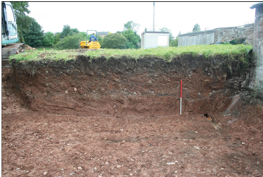
Plate 7: Section showing the depths of the natural clay ( 102 ) and subsoil ( 101 ), following wall removal on the east side of the site (looking west).
