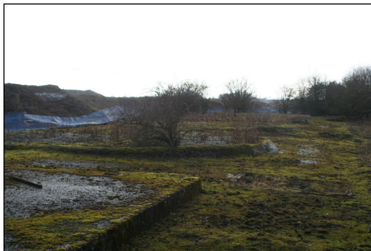
Plate 17. Concrete fuel tanks (Structure 16) on the northwest side of the survey area looking southeast.
