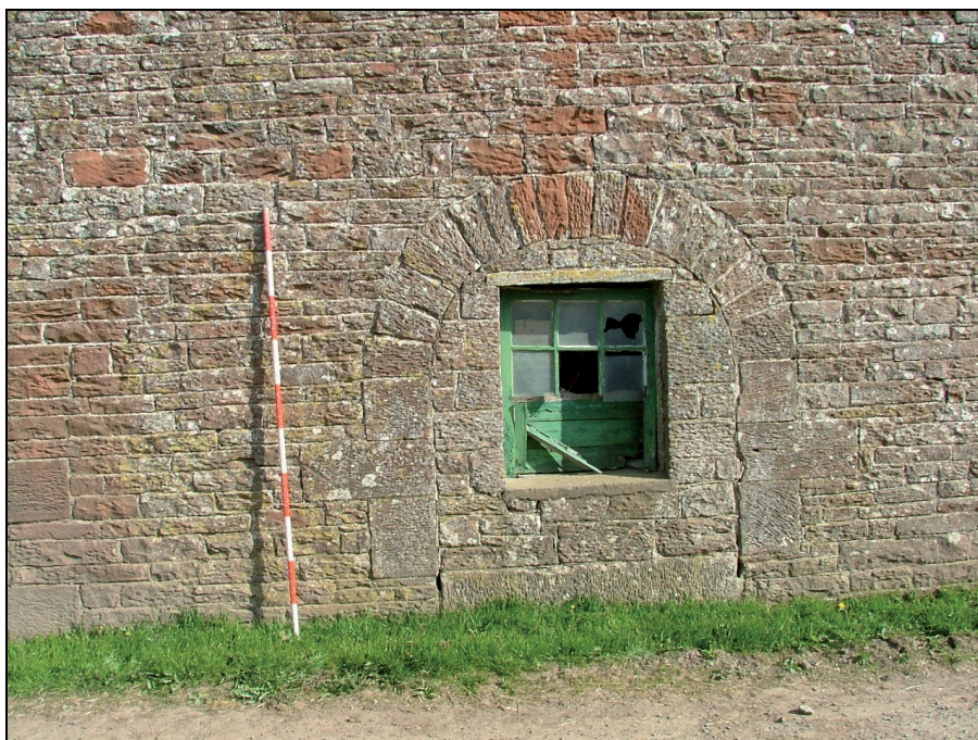
Plate 39: Detail of one of the blocked arched doorways with inserted window, south elevation of Building A (Scale = 2m)
