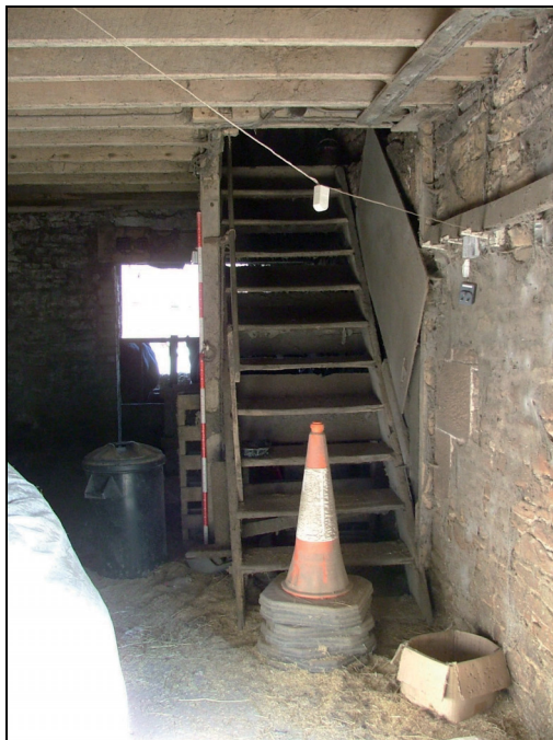
Plate 41: Detail of wooden staircase to first floor of Building A (Scale = 2m)
