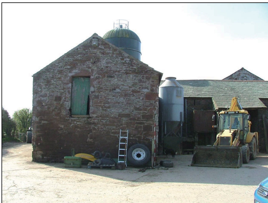
Plate 12: View looking south showing the north gable, with the barn to the right of photograph (Scale = 2m)
