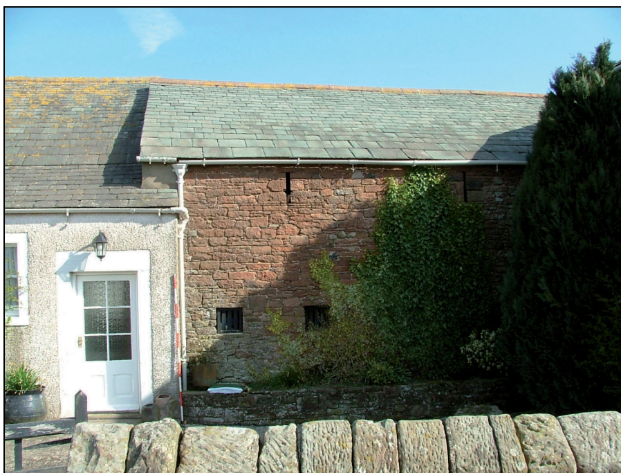
Plate 30: Part of the south elevation of the barn, showing two small windows (Scale = 2m)
