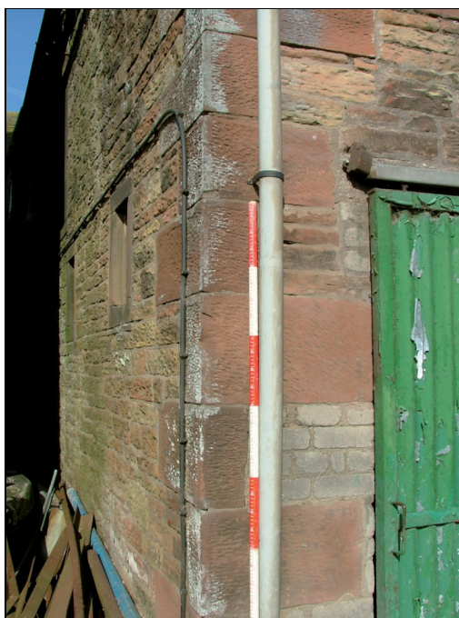
Plate 5: Detail of the alternating quoins consisting of well-dressed masonry blocks of sandstone at the corner of the east and south elevations
