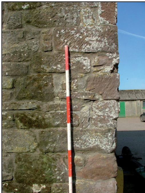
Plate 6: Detail of the quoins at the corner of the east and north elevations
