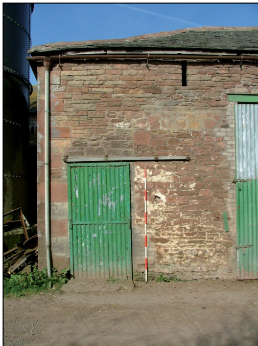
Plate 4: Detail of the vertical construction break in the east elevation showing the well dressed quoins of the addition to the south (Scale = 2m)
