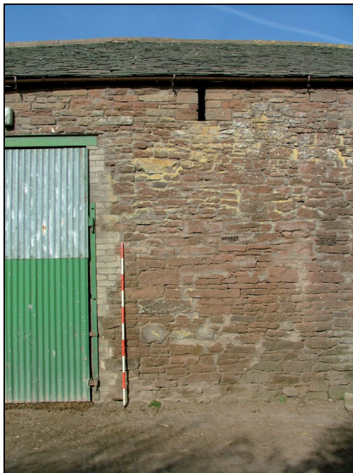
Plate 8: Detail of vertical break in the masonry of the east elevation to the north of the inserted doorway (Scale = 2m)
