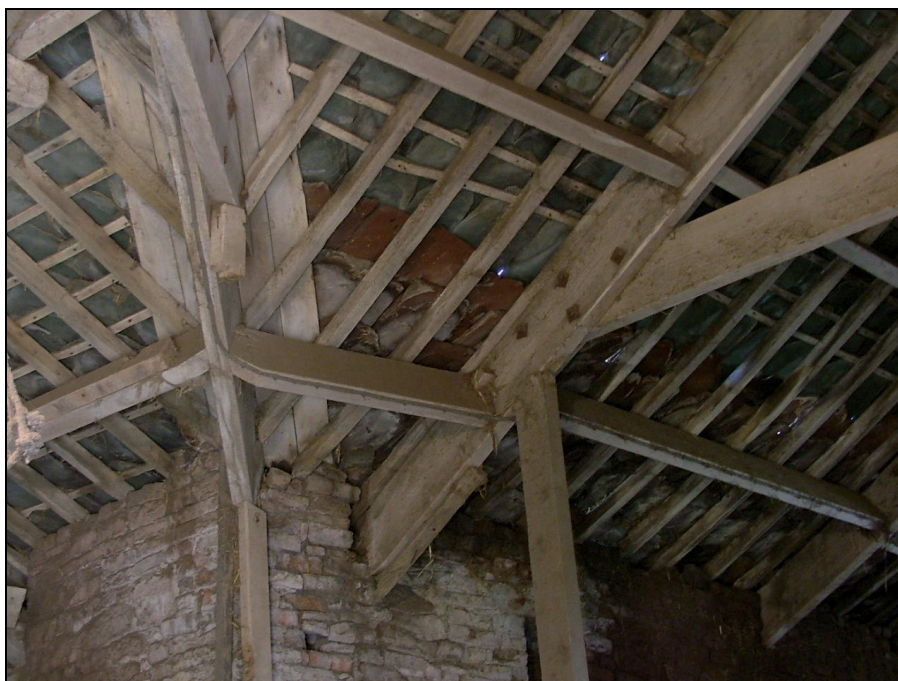
Plate 25: Detail of the roof structure at the 90° angle between the survey building and the barn
