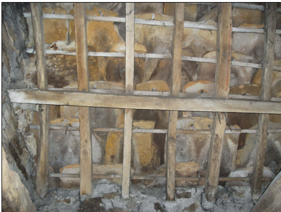
Plate 57: Detail of the underside of the stone slate roof showing the wooden pegs used to hold the slates in place
