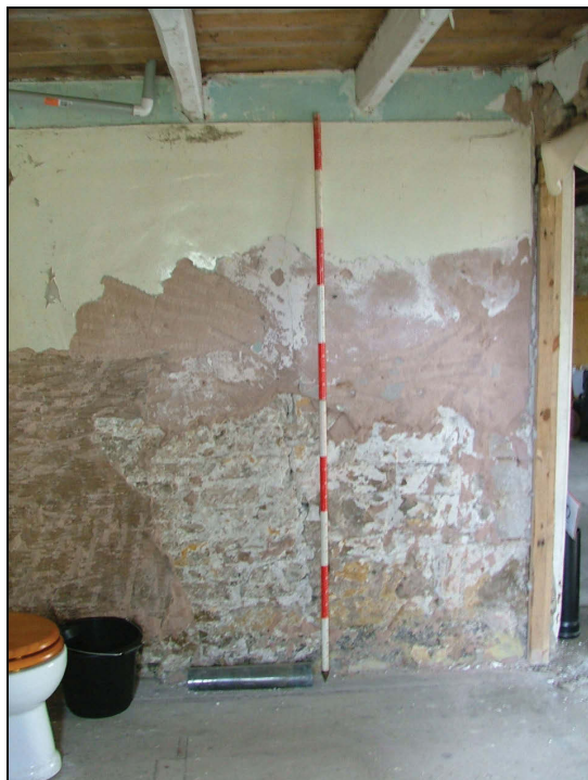
Plate 45: North-west wall of the ground floor bathroom showing the possible vertical break of a former doorway (Scale = 2m)
