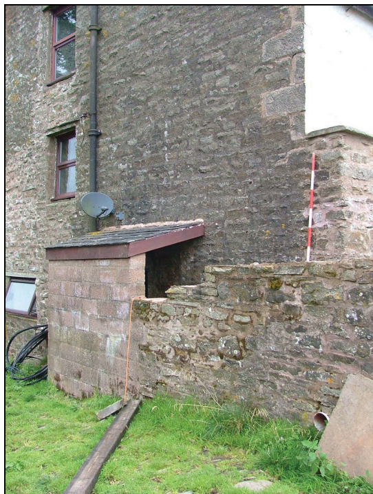
Plate 22: Detail of the modern porch for the doorway in the south-west elevation
