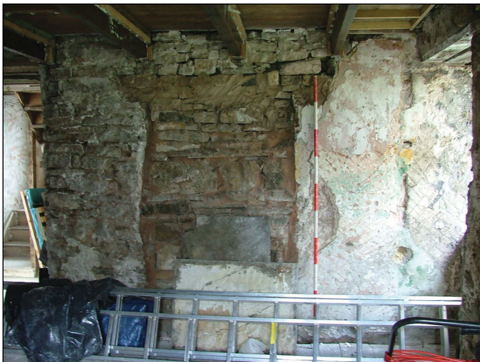
Plate 39: Possible former cupboard or shelf recess, south-east wall of Reception Room 1 (Scale = 2m)
