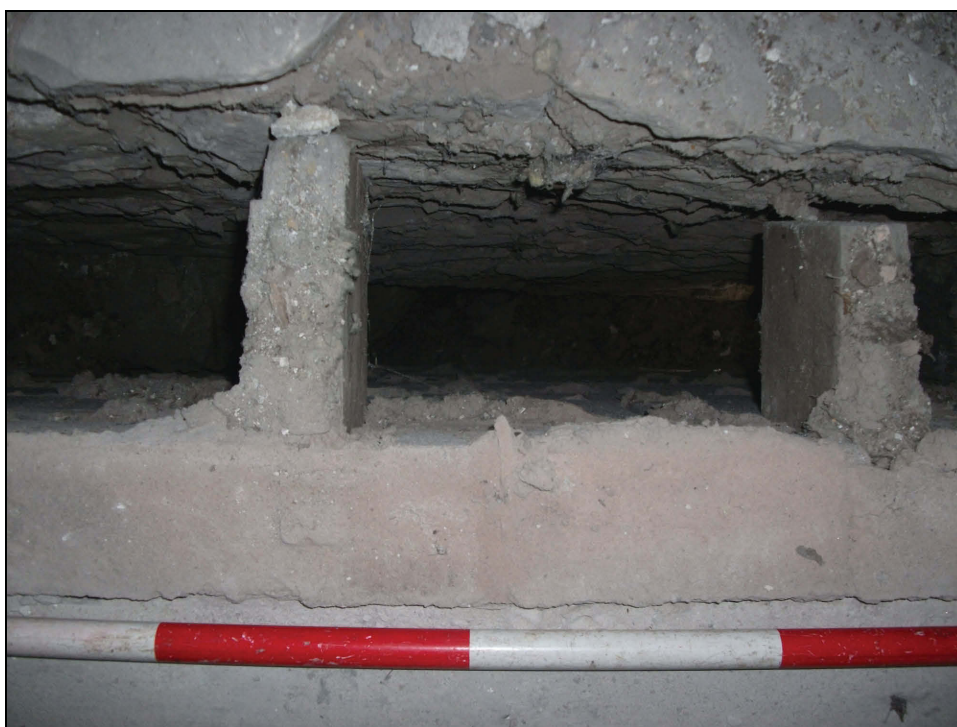
Plate 60: Detail of the gap between the blockwork of the ground floor room and the inner face of the masonry wall, as seen from first floor Bedroom 2
