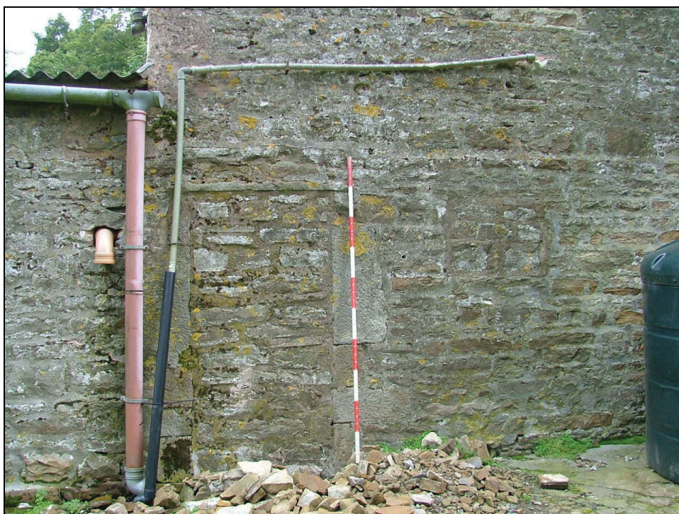
Plate 29: View looking north-east showing blocked door and window in the south-west wall of the southern outshut (Scale = 2m)
