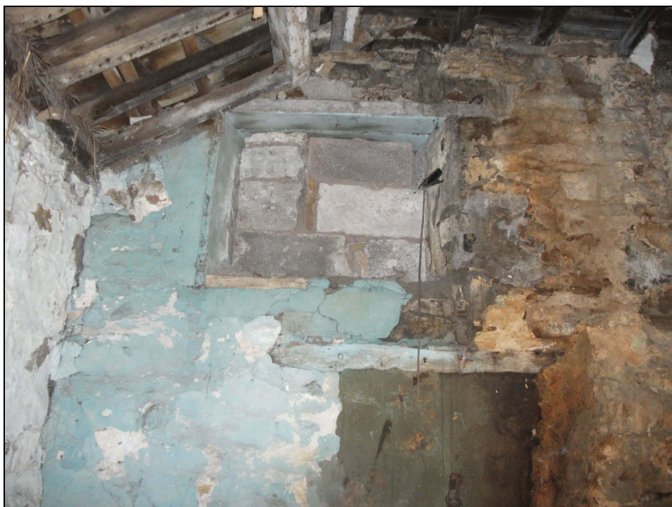
Plate 63: Detail of two blocked windows to the left of the chimney breast, Bedroom 2
