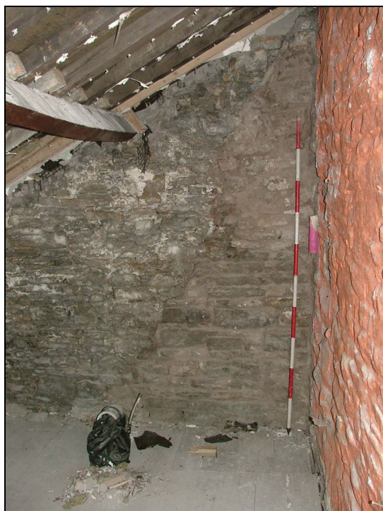
Plate 48: South-west wall of upper room in outshut showing changes in the masonry, possibly simply an area of repointing (Scale = 2m)
