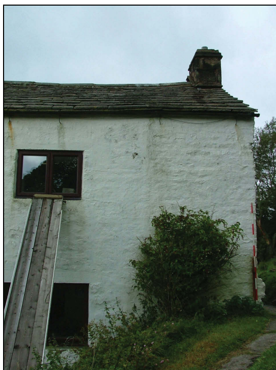
Plate 15: Blocked window beneath the eaves, north end of the south-east elevation (Scale = 2m)
