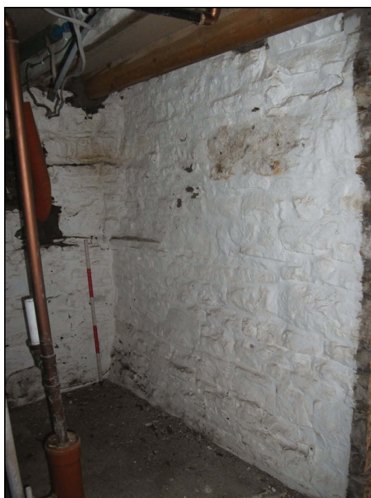
Plate 72: South-west wall of Room 1 in the basement with the remains of stone shelves visible in the corner (Scale = 1m)
