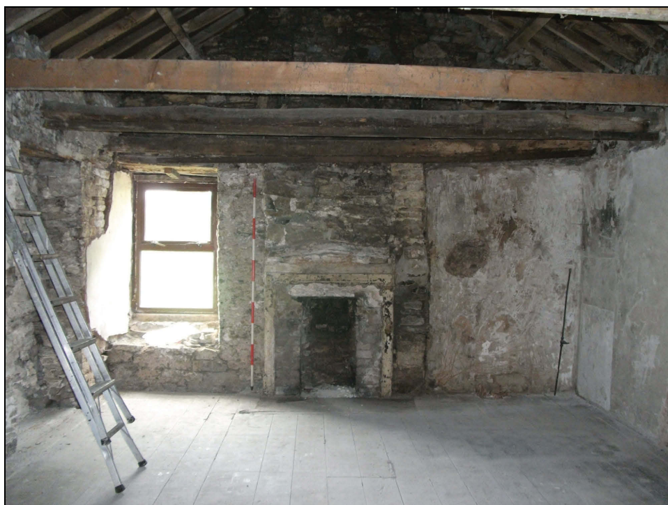
Plate 50: South-west internal wall of Bedroom 1 (Scale = 2m)
