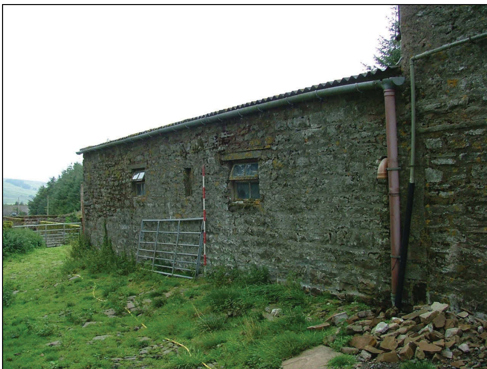
Plate 31: The single-storey farm building (former byre) to the north-west side of the house
