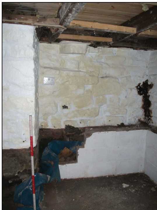
Plate 73: North-east wall of Room 3 in the basement showing a corbel which supports the fireplace above (Scale = 1m)
