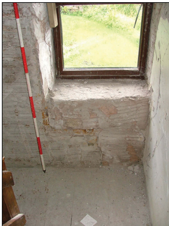
Plate 47: Base of the staircase window showing it was formerly a larger aperture
