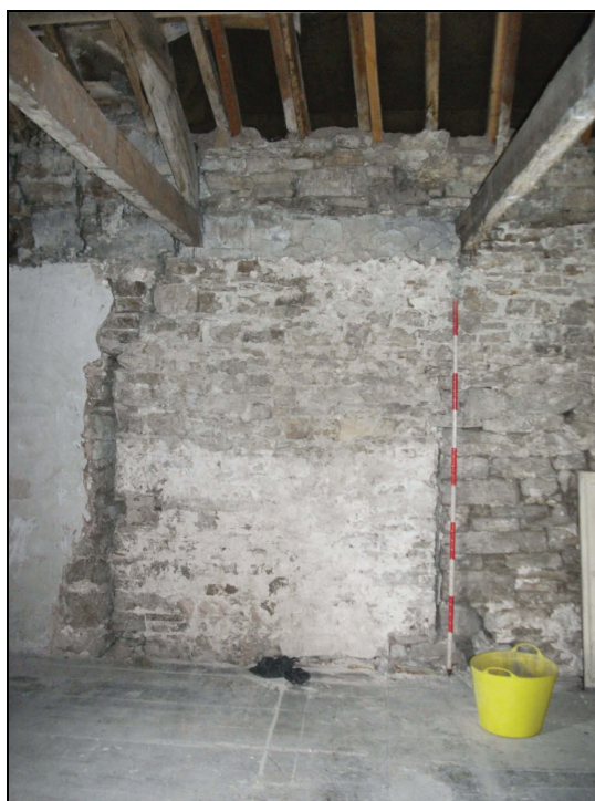
Plate 53: North-west wall of Bedroom 1 showing disturbance in the masonry (Scale = 2m)
