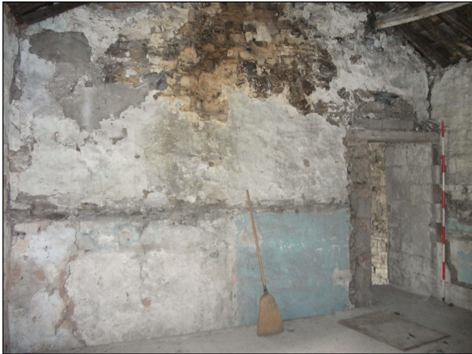
Plate 69: South-west elevation of Bedroom 2 showing the horizontal line of a former floor level and the inserted doorway (Scale = 2m)
