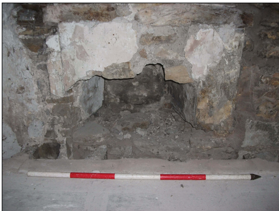
Plate 67: Detail of former window in south-east wall of Bedroom 2, showing the splayed reveals and remains of plaster (Scale = 1m)
