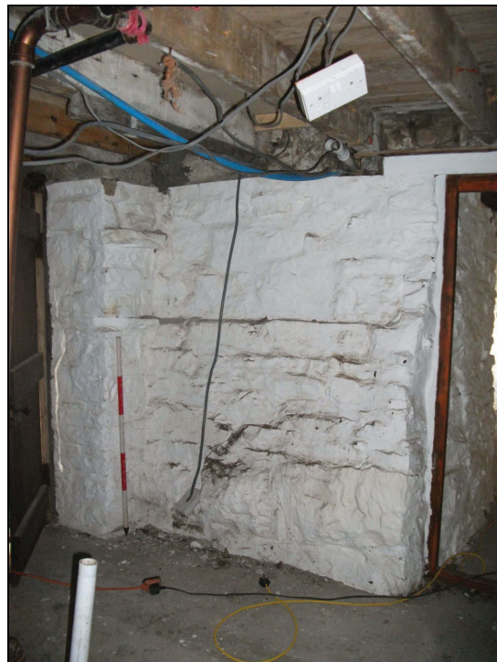
Plate 70: North-west wall of Room 1 in the basement displaying evidence for former stone shelves (Scale = 1m)
