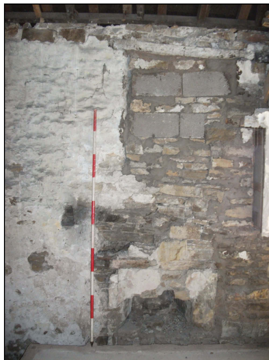
Plate 66: South-east wall of Bedroom 2 showing two blocked windows, one just below eaves level, and the other at present floor level (Scale = 2m)
