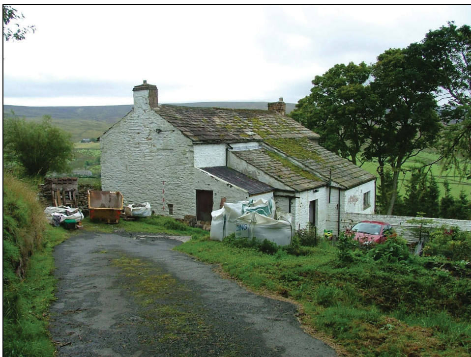
Plate 5: View looking south from the access track showing the north-east gable and the north-west elevation of High Scilly Hall
