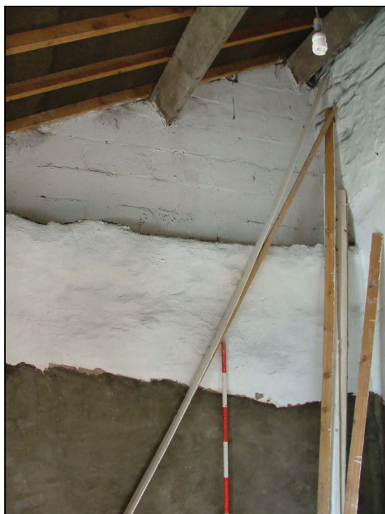
Plate 34: Detail of modern blockwork used to create the pitched roof of the outshut which houses the vestibule
