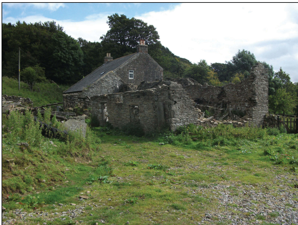
Plate 77: View looking east showing the renovated house at Low Scilly Hall and the ruined farm buildings to the western side
