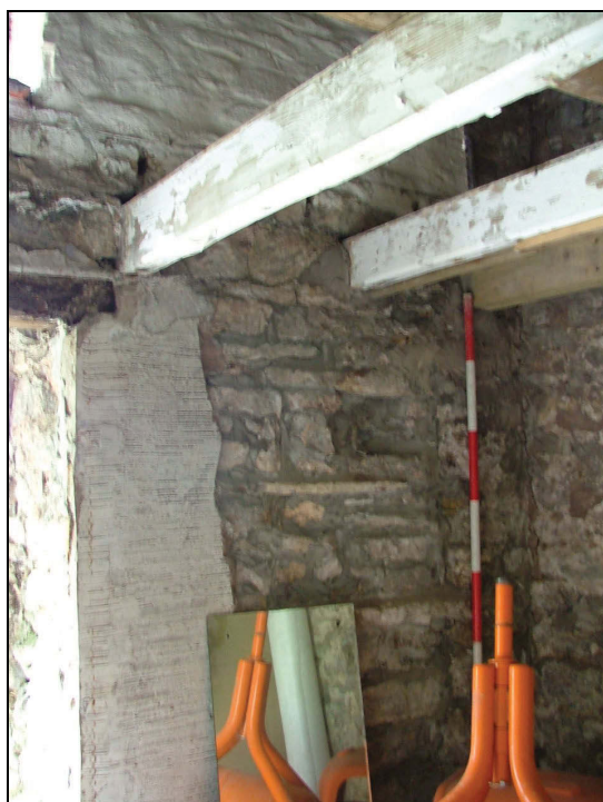
Plate 44: Blocked opening, possibly a former window, but which contains evidence for shelving, ground floor bathroom
