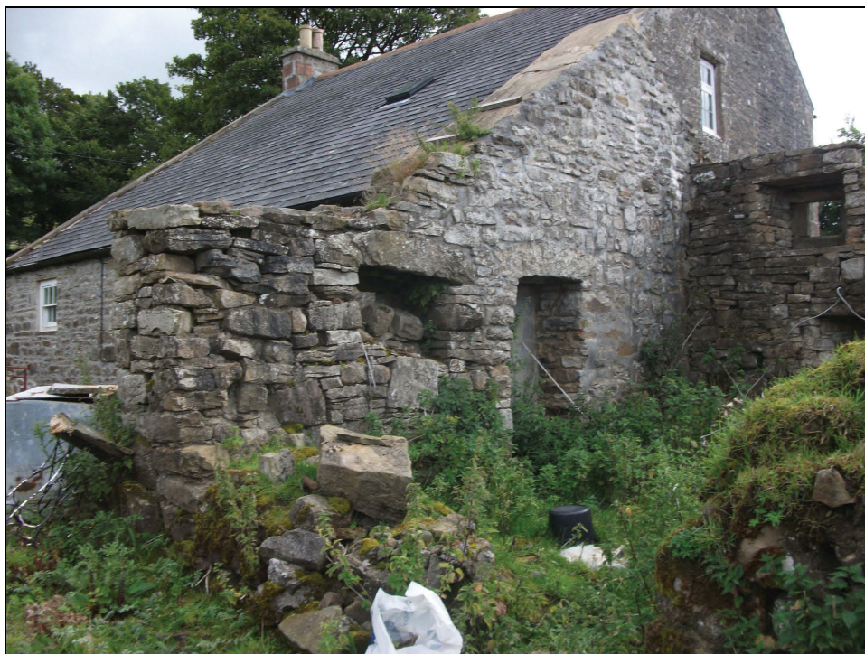
Plate 80: Detail of part of the ruined buildings at Low Scilly Hall, possible bastle or tower house
