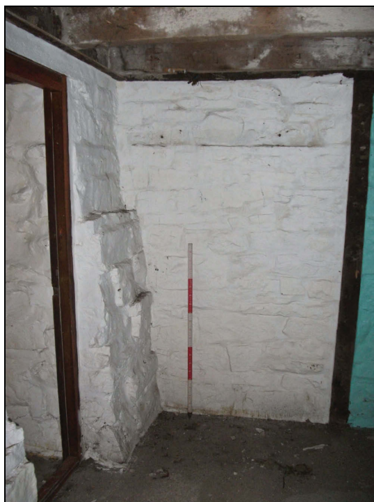
Plate 71: North-east wall of Room 1 in the basement showing the remains of former stone shelves (Scale = 1m)
