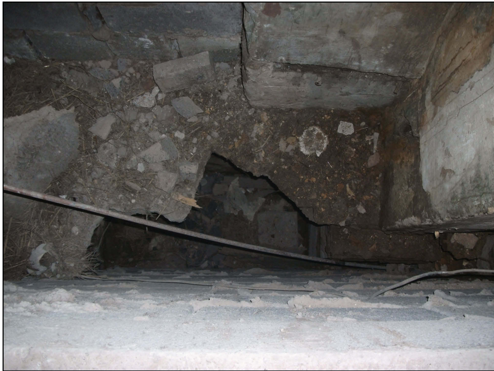
Plate 65: View looking down the gap between the blockwork and masonry wall, as seen from Bedroom 2, showing a further room below that which was heated by the large fireplace shown on Plate 61
