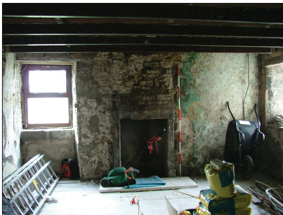
Plate 36: Fireplace in the south-west wall of Reception Room 1, ground floor (Scale = 2m)
