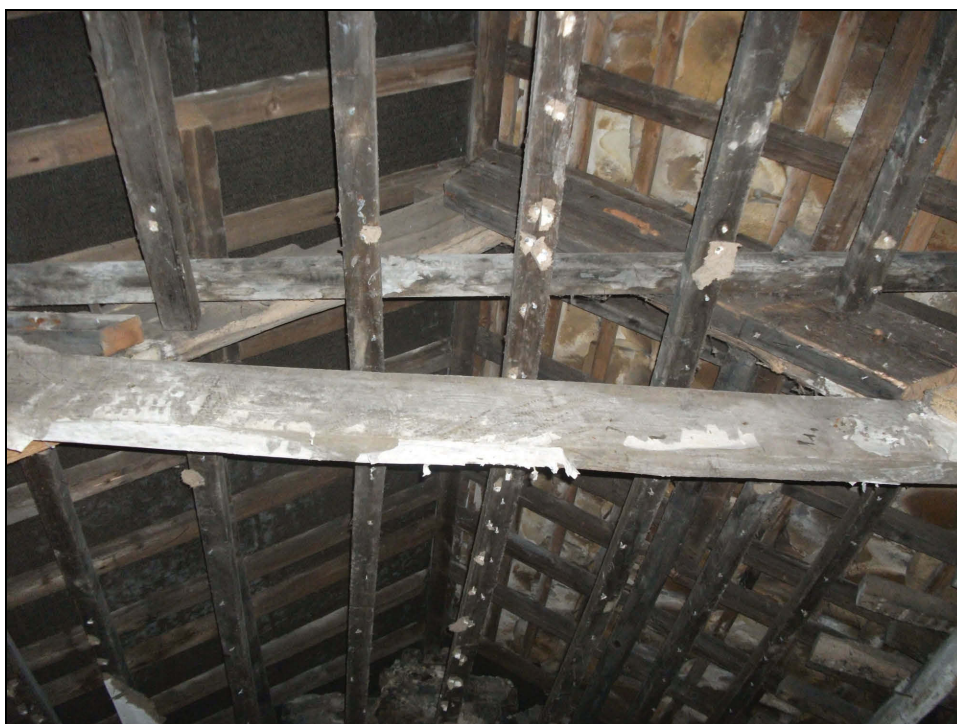
Plate 59: Detail of the timber work to which the former ceiling was fixed, Bedroom 2
