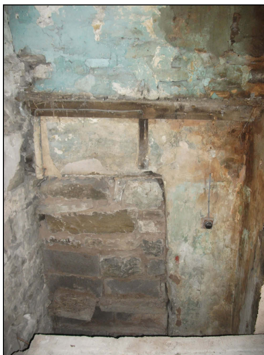
Plate 64: Blocked doorway to left hand side of chimney breast, as seen from Bedroom 2
