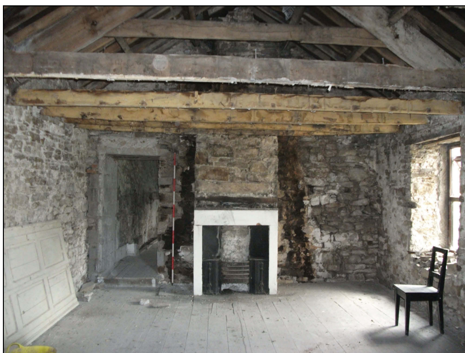
Plate 54: North-east wall of Bedroom 1 showing the central fireplace and smoke- marked wall of a possible earlier flue (Scale = 2m)
