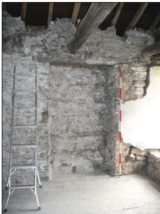
Plate 49: South-east wall of Bedroom 1 showing the recess for a cupboard or shelving (Scale = 2m)
