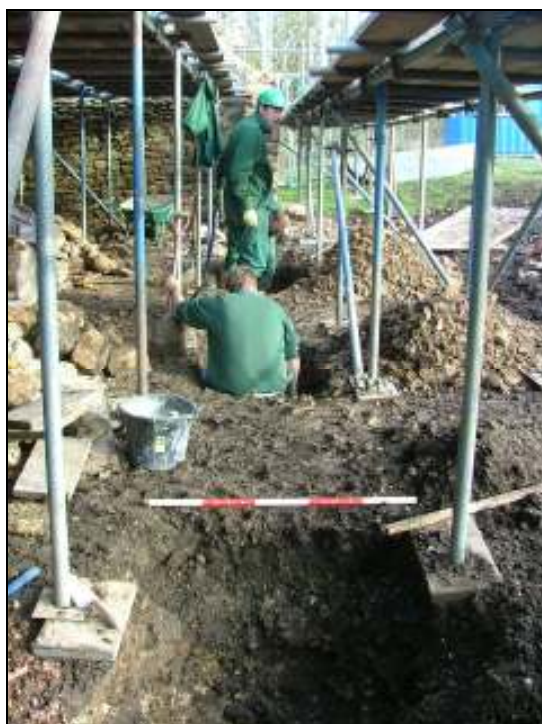
Plate 3: View looking east showing the excavation of the three foundation holes along the line of the south elevation of The Hemmel (November 2010)
