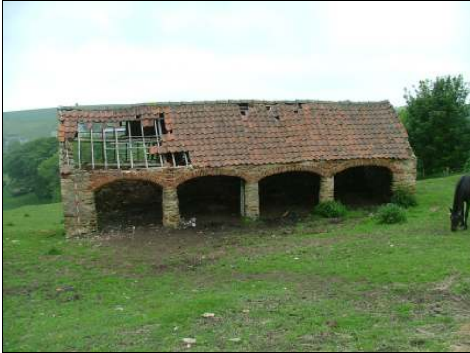
Plate 1: South elevation of The Hemmel showing the three piers as they existed in June 2010 prior to restoration work
