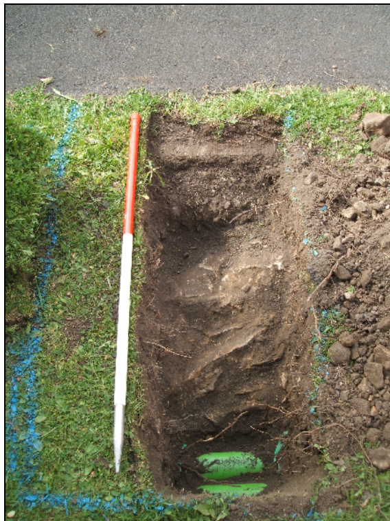
Plate 8: Foundations (115) to the west of excavated area, Avalon Drive, Denton Burn, looking southwest
