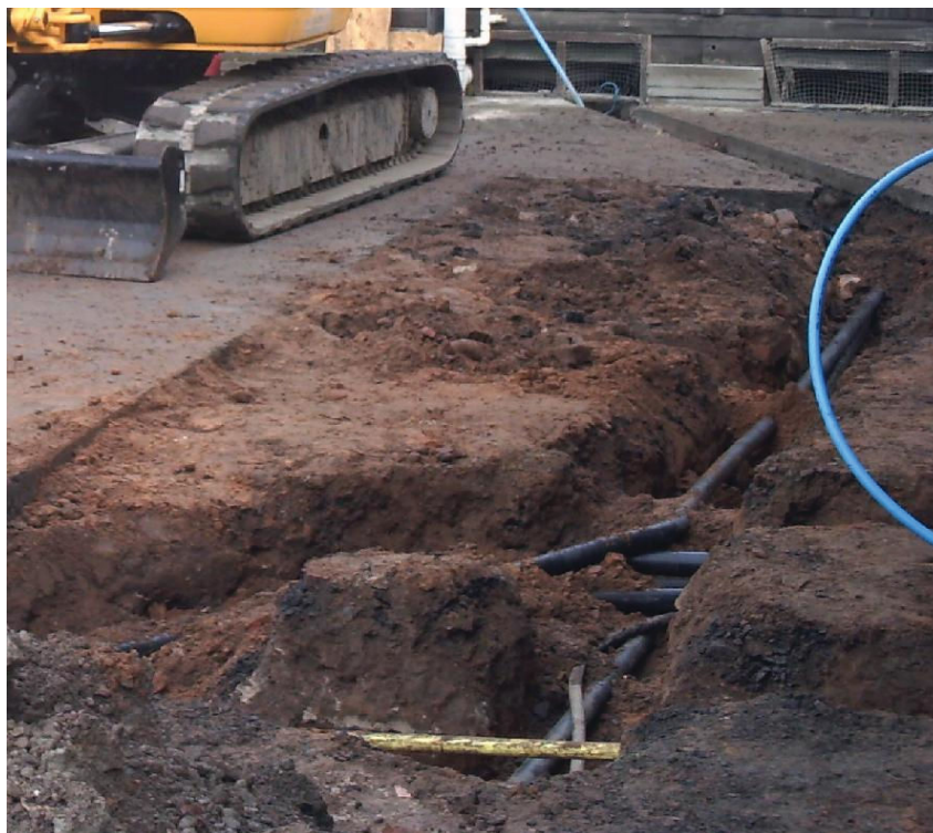
Plate 3: Shot of Trench 1 (foreground), Trench 3 (right side & background) and Trench 4 (lower centre, behind Trench 1), looking NE
