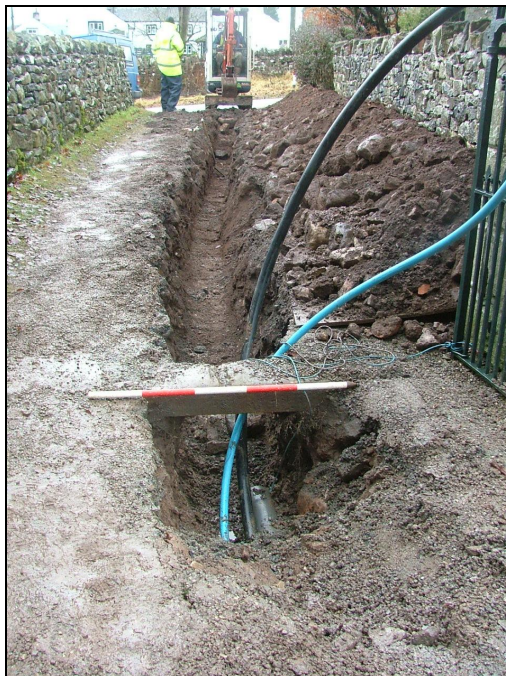
Plate 21: View looking west showing the excavation of the trench from the church gates towards the road (Scale = 1m)
