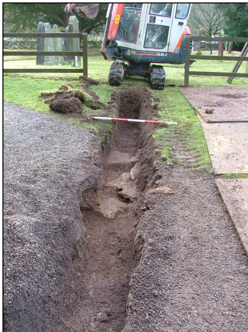
Plate 29: View looking south showing the remains of a wall (112) within the drainage trench (Scale = 1m)
