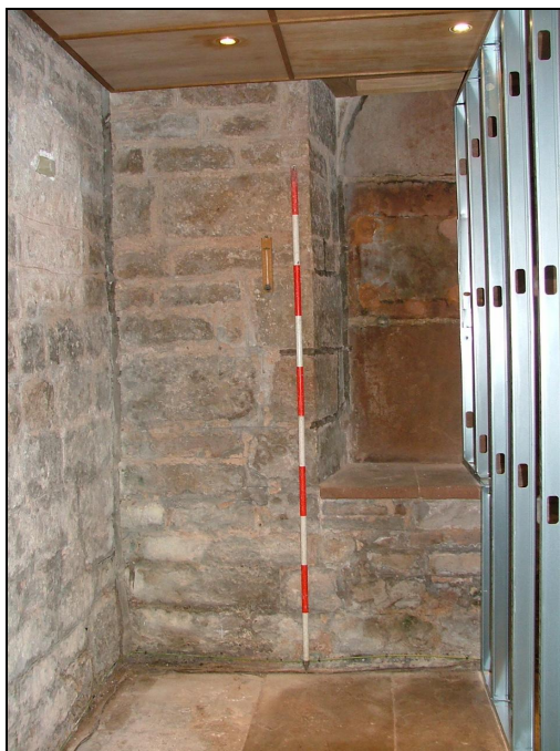
Plate 33: Interior of the north wall where the toilet is to be located (Scale = 2m)
