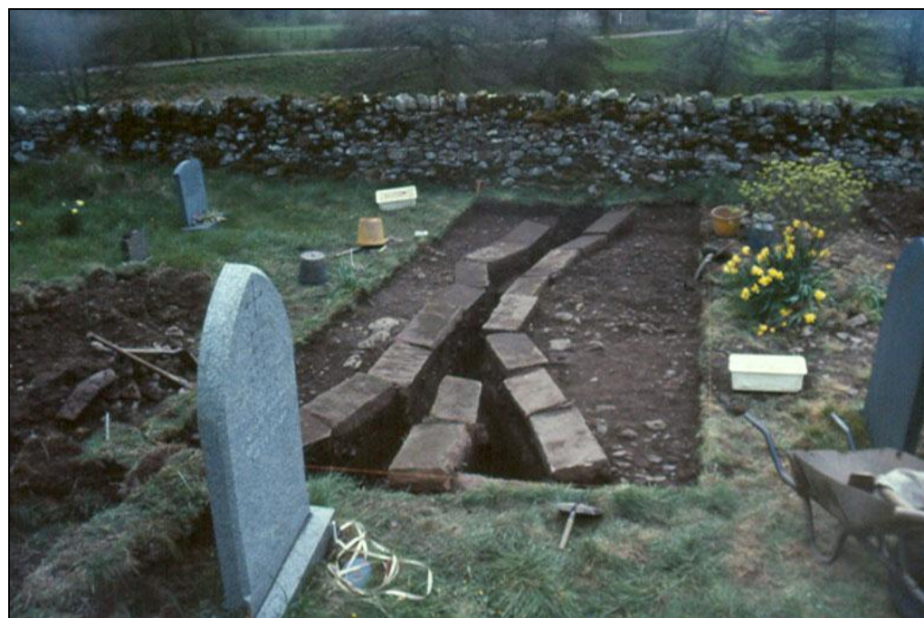
Plate 4: View looking south of the re-excavated drain in the 1980s (Courtesy of Alan James)
