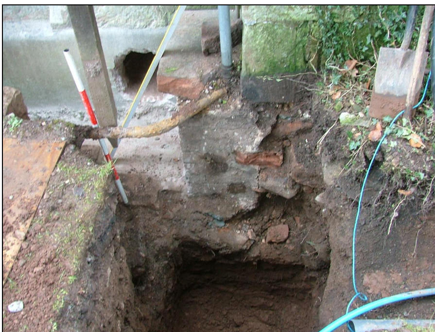
Plate 26: View looking south showing the trench for the 2m high pump chamber (Scale = 1m)
