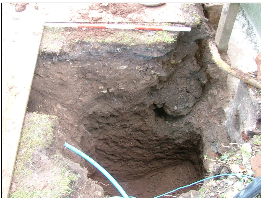
Plate 25: View looking east showing the trench for the pump chamber. The collapsed remains of a stone culvert are visible to right of photograph (Scale = 1m)
