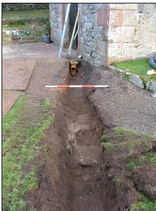
Plate 28: View looking north showing the drainage trench leading off from the south-west corner of the church tower, with the remains of a wall visible within the trench (Scale = 1m)
