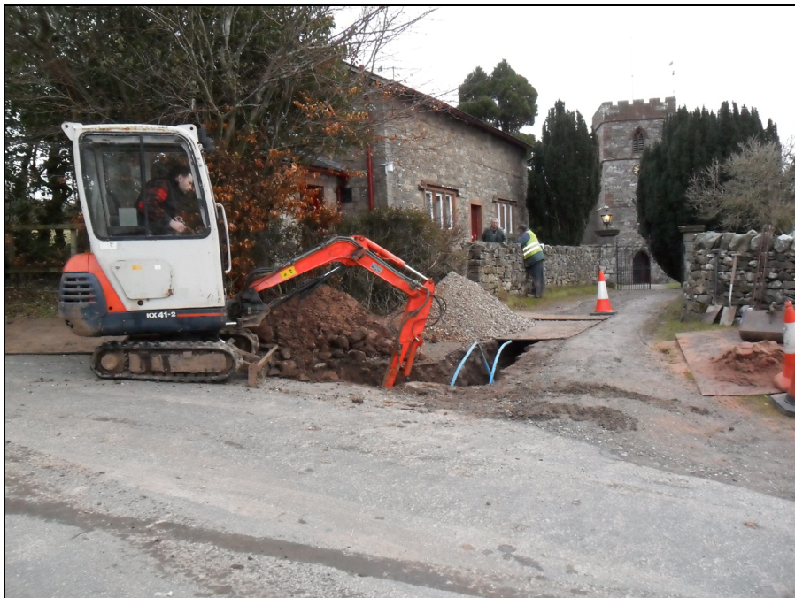
Plate 23: View looking east showing the excavation of trenches to the west of the church
