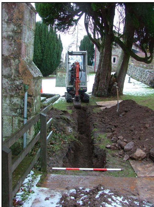
Plate 15: View looking west showing the excavation of the service trench from the north-west corner of the church in a westerly direction (Scale = 1m)
