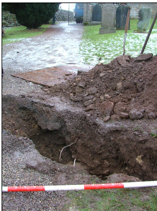
Plate 18: View looking west showing the point where the trench reaches the gravel path. The remains of a stone wall or culvert were noted in the trench
