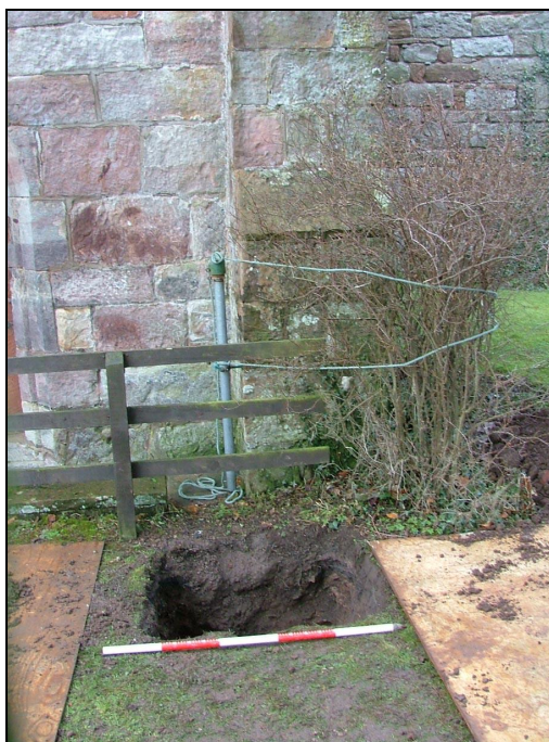
Plate 12: View looking south showing the location for the pump chamber (Scale = 1m)
