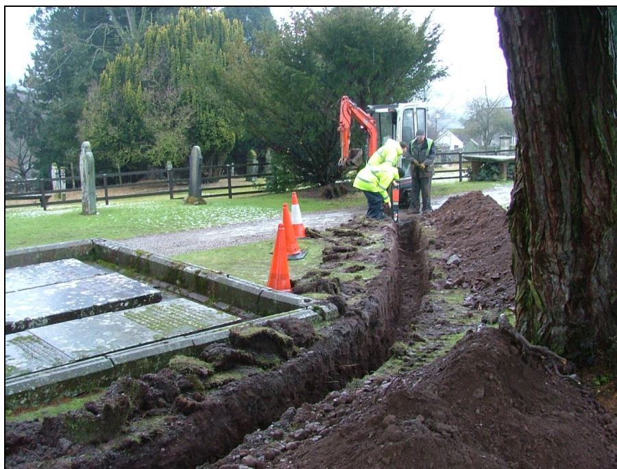
Plate 17: View looking south-west showing the route of the service trench up to the pathway to the west of the church
