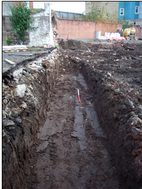
Plate 2: Boundary Wall Foundation Trench, South West Corner of the Site (facing north)
