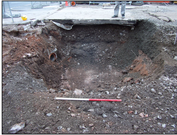
Plate 10: Stratigraphy at the Eastern End of the Site after the Removal of a Large Manhole (facing south)
