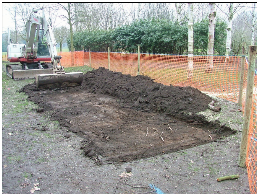
Plate 2: Eastern end of the footpath route showing the width and depth of the trench
