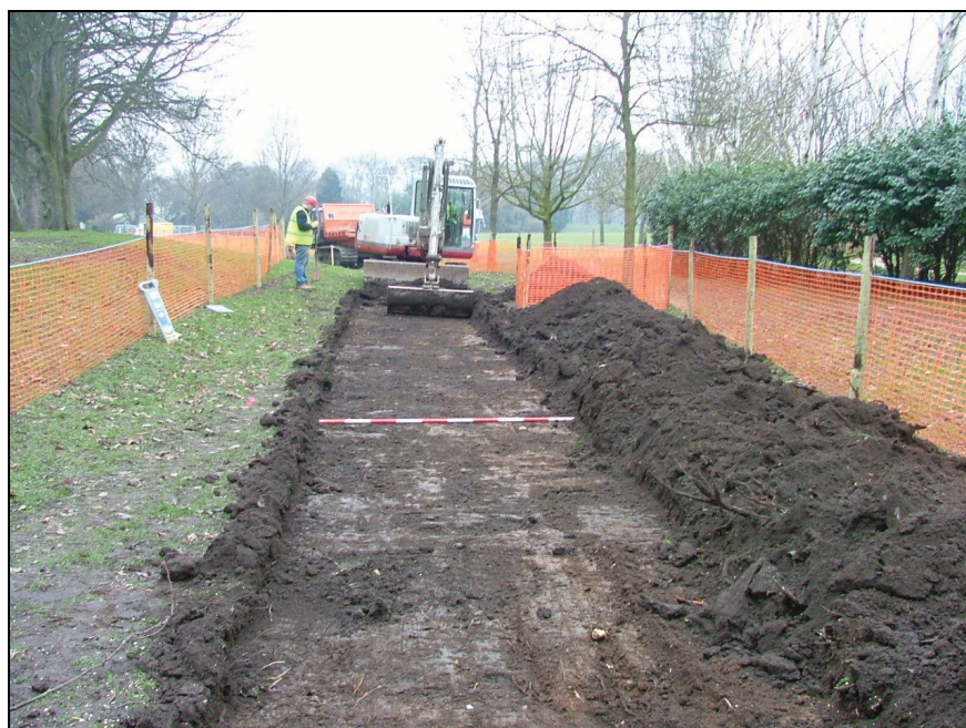
Plate 3: View looking west showing the eastern end of the excavated trench (Scale = 2m)
