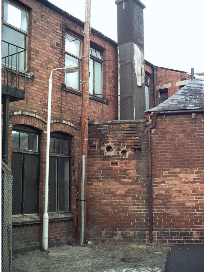
Plate 3: Western corner between main northern block and eastern wing. (Taken from alley running to the rear or Richardson Street)
