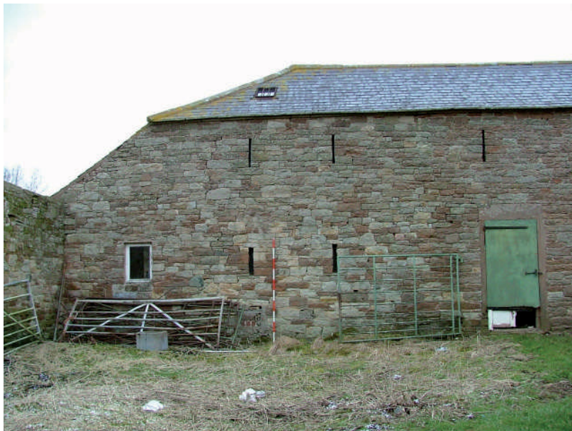
Plate 3 – South facing elevation of Barn A, showing outshut on western elevation is contemporary with the rest of the building
