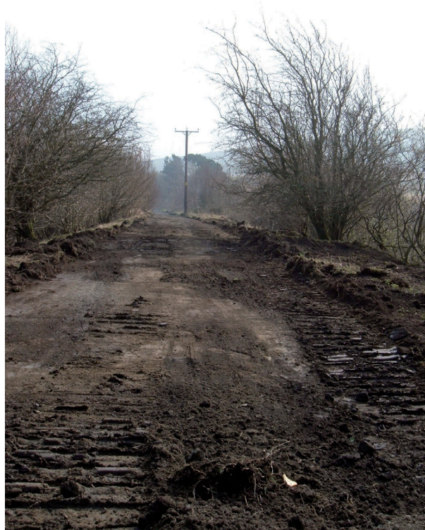
Plate 2: The stripped cyclepath on the embankment west of Rose Cottage
