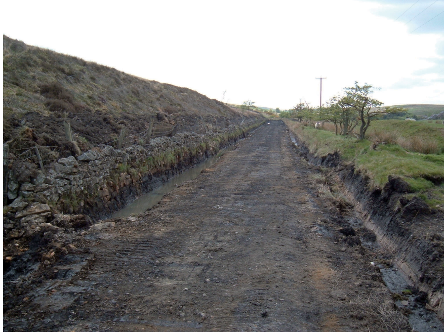
Plate 7: The formerly wet area west of Prior High Side Drift after stripping for cyclepath and excavation of new drainage ditches
