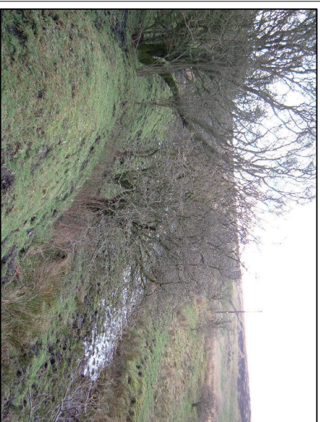
The cutting just west of Whites Cut, note the waterlogged state of the trackbed
