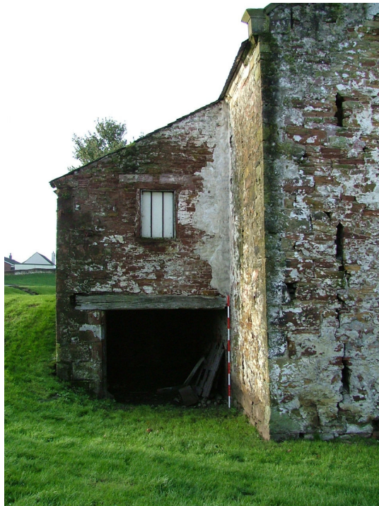
Plate 5 – North-east facing elevation of bank barn showing large doorway and upper window of outshut
