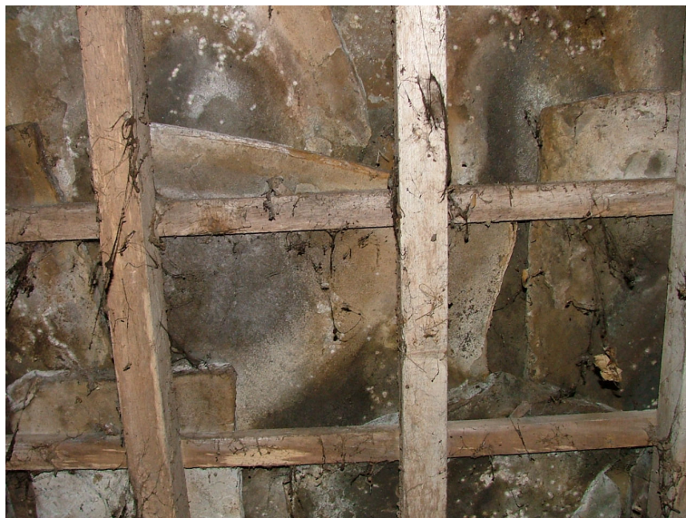
Plate 7 – Interior of roof above hayloft showing stone tiles with wooden pegs resting on the laths
