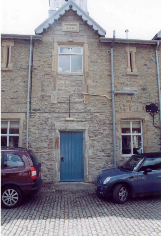
Plate 12: View of central bay of north facing elevation of central range, illustrating reduction in size of window
