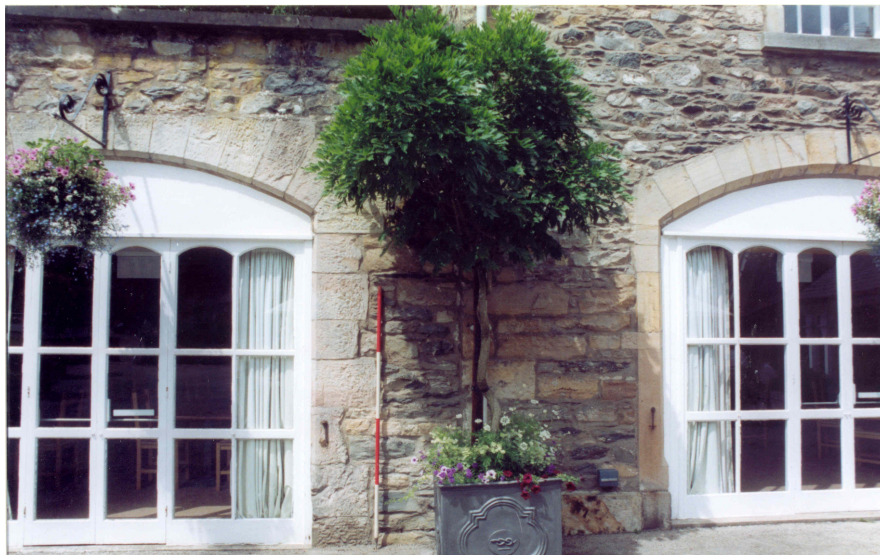
Plate 3: Detail of straight joint between later extension and primary Stable Block: Internal elevation looking North-W
