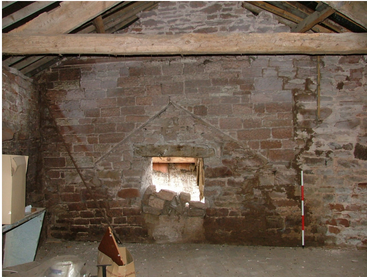
Plate 28 – Scarring of an earlier building in the southern gable end of Range C
