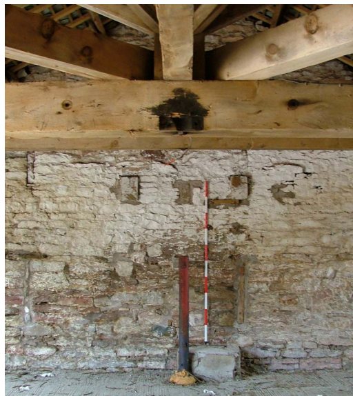
Plate 9 – Timber stumps and blocked hole, gin-gang
