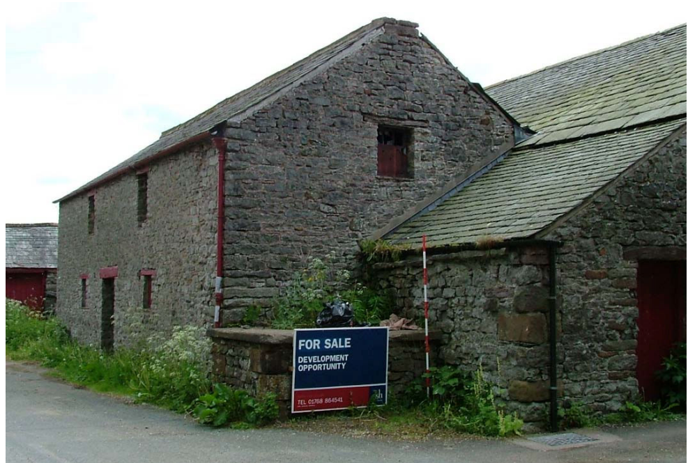
Plate 11 – SW facing elevation of Building 3, showing window and remains of chimney stack
