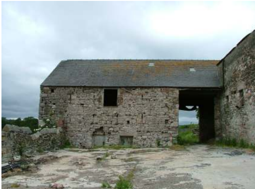
Plate 12: South East facing elevation of Barn B, showing large doorway, two small apertures at ground level and pitching door at first floor level
