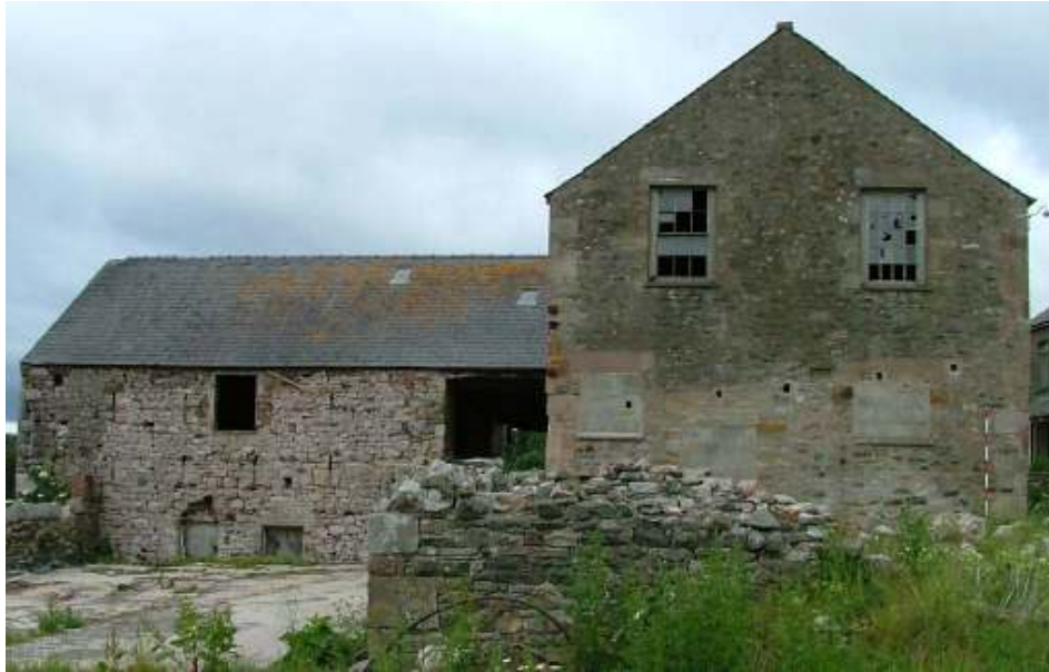
Plate 15: South facing gable end of Building 4, with the western end of Barn B
