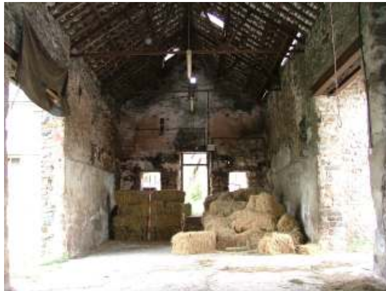
Plate 13: North East gable end of Barn B, the joist holes for first floor are just above the plaster line.
