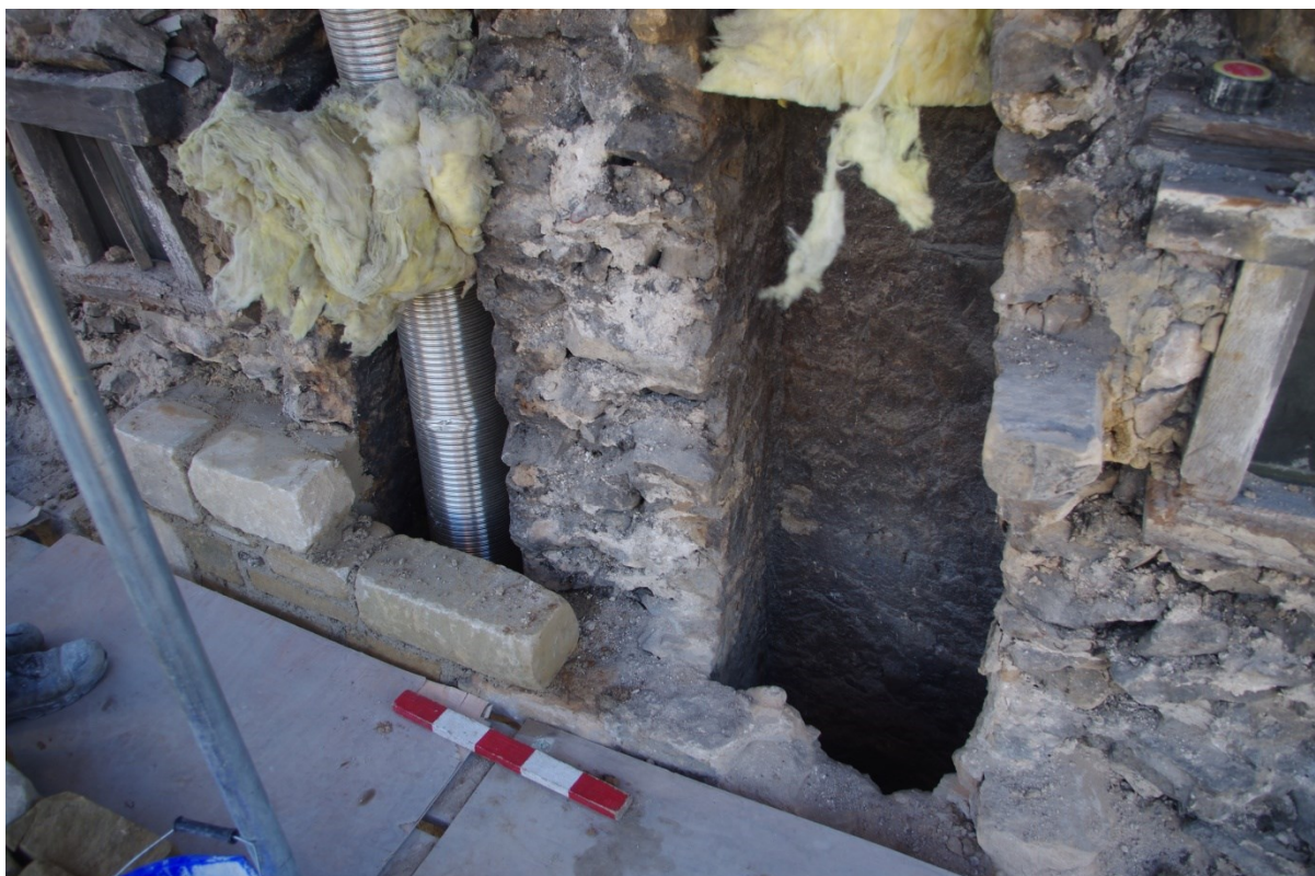
(11) The twin flues of the chimney revealed by the removal of the outer wall face.
