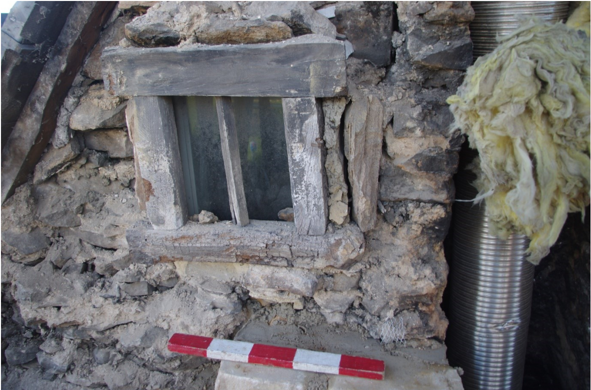
(12) The eastern upper window in the north gable end, with timber frames revealed when the outer face of the wall was removed
