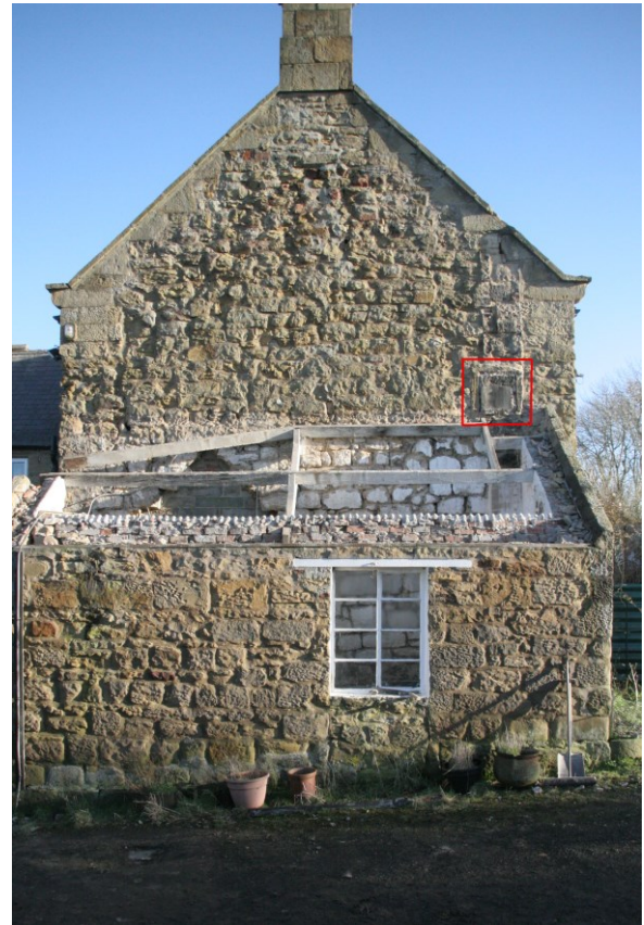
West gable end; new opening just visible (left) above wall of roofless Wash House; to right (outlined in red) is original first-floor window exposed by removal of stack (see front cover for enlarged view)
