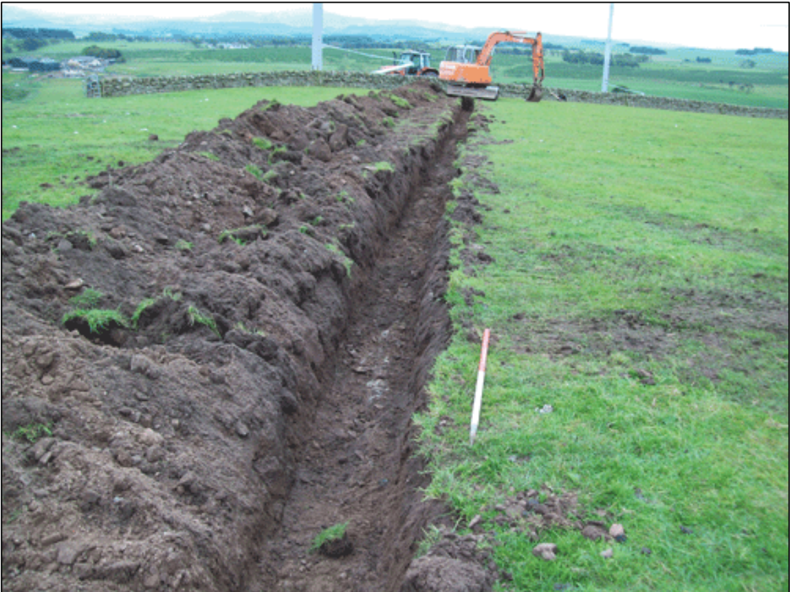
Figure 4b: Cable trench from the north
