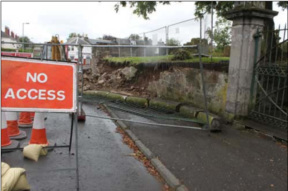
Figure 5b: General View from west, following collapse of Retaining Wall 000
