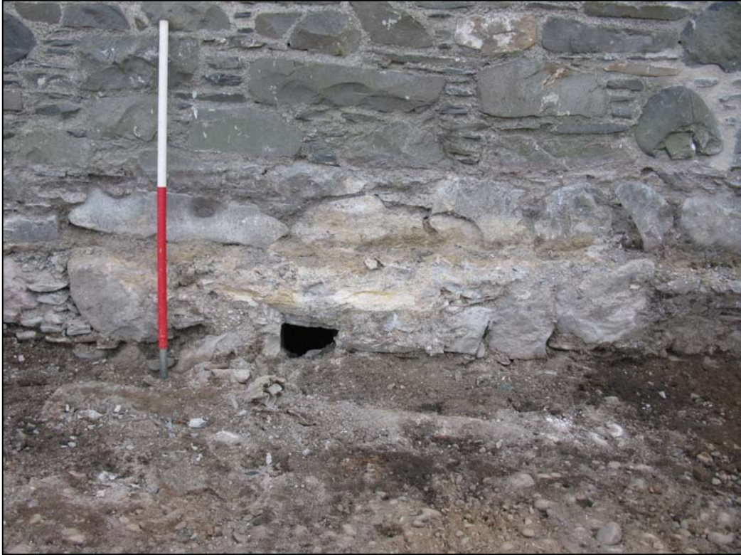
Figure 7a: In Situ ? Drain (011) in W-Facing Elevation of Castle
