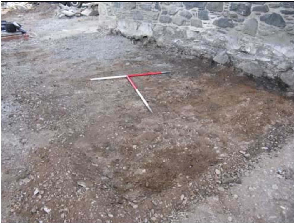
Figure 7b: Surface cleaned, N Side (W Facing Elevation), with Foundation Trench [014]/(015) visible
