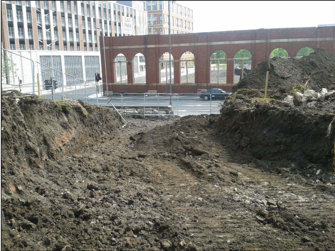
Figure 3a: Demonstrating deposits (001) & (002) within access road
