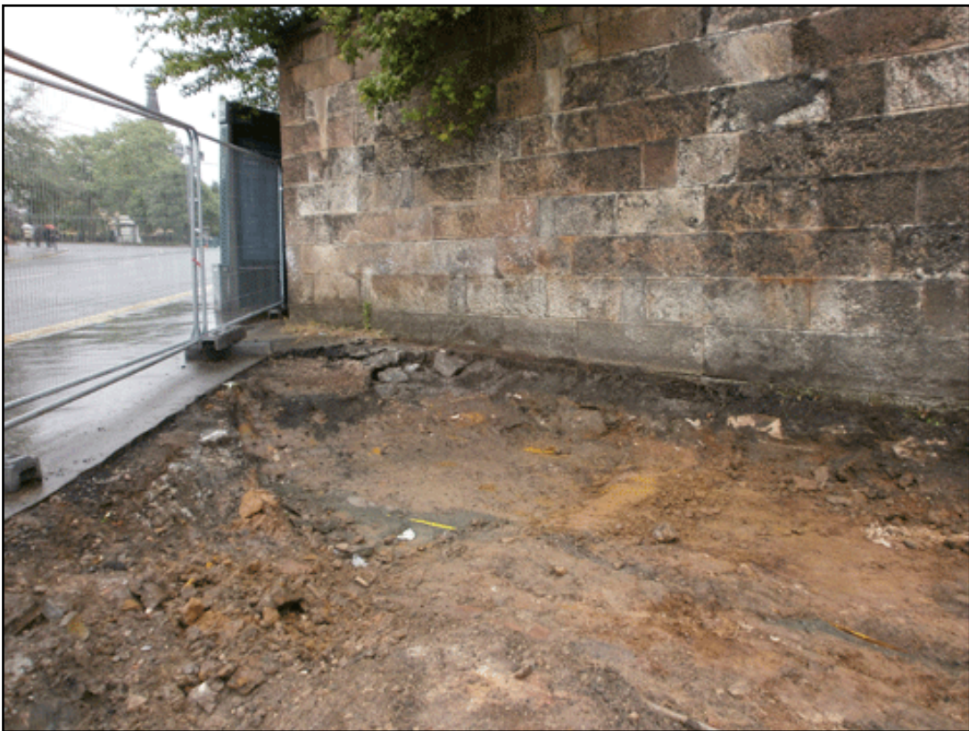
Figure 3b: Subsoil (012) at west side of Prison Wall [022]
