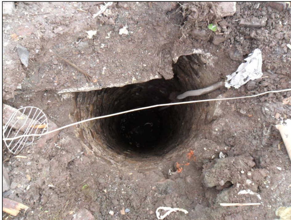
Figure 3b: The well discovered during demolition and part of the sandstone cap to the top of the photo
