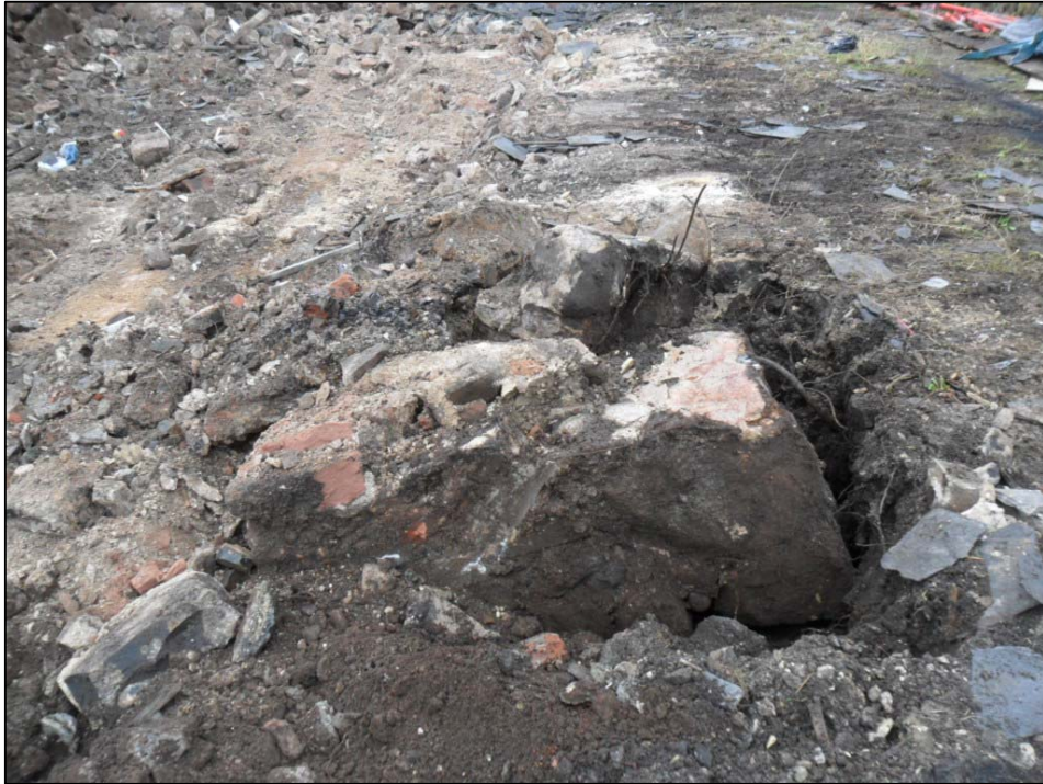
Figure 4a: Remains of foundation from the western wall of the Stevenson Institute
