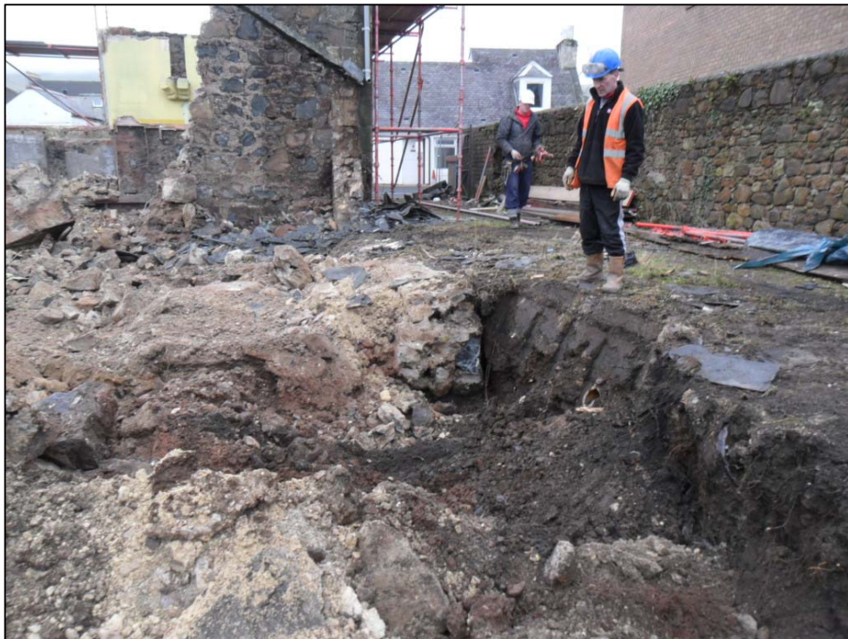
Figure 4b: Showing the depth of the foundations removed along the southern edge
