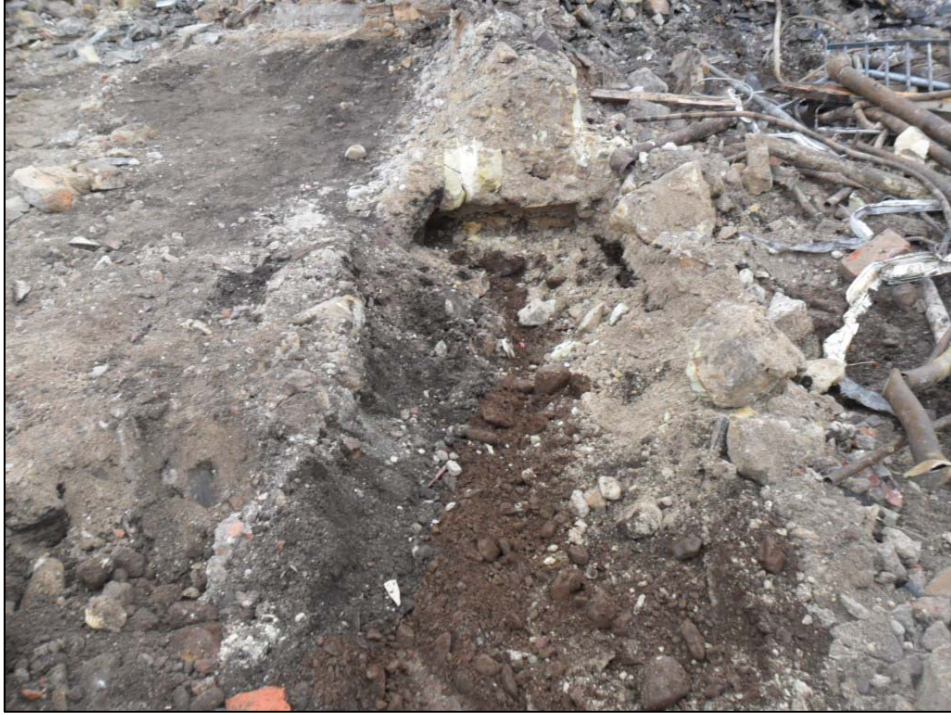
Figure 5: Demonstrating the shallow depth of the foundations sitting directly on to (002) and forming the rectangular structure.
