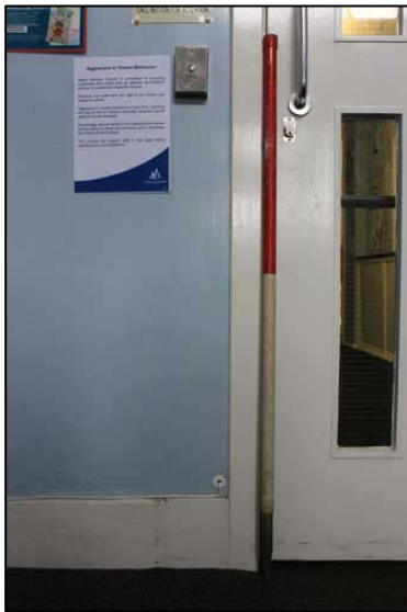
Fig. 10c: Room a, Altered Skirting
