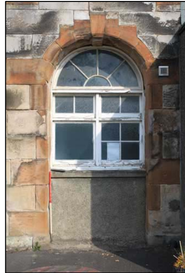
Fig. 8b: Industrial School, E Elevation, Blocked Entrance
