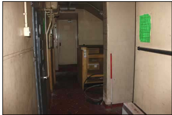
Fig. 8d: Cable Moulding & Bar Area
