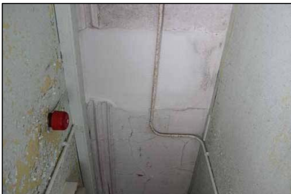
Fig. 6e: Room i, Break in Cornice
