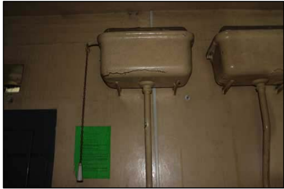
Fig. 8a: Wall-Mounted Cistern Outside Cell
