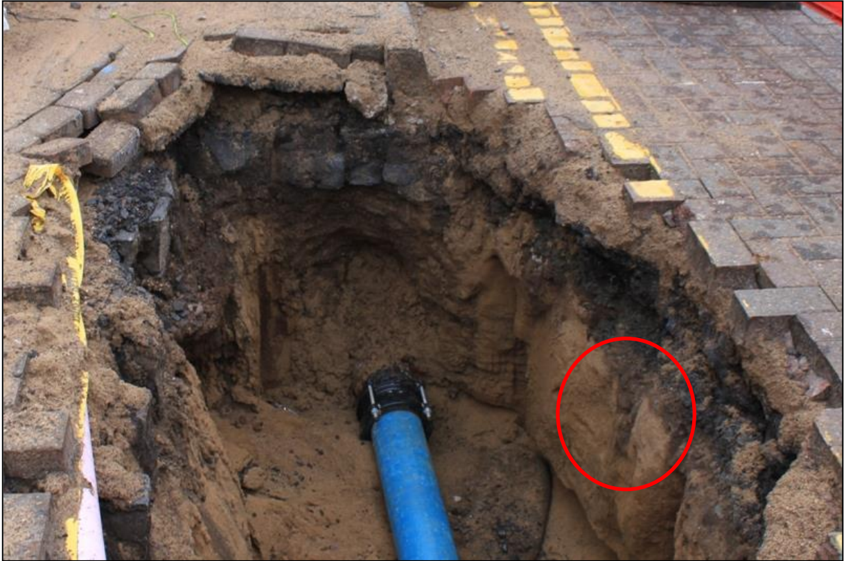
Figure 3a: Eastern pit of Scottish Water works outside the Townhouse (H) with nineteenth century cobbled surface visible underneath modern pavement.
