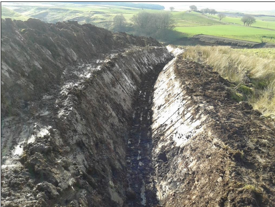
Figure 4b: Eastern stretch of the cable trench near the sub-station at Ardoch from the east.
