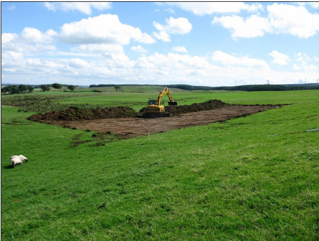
Figure 5b: Post excavation view of compound strip at Over Enoch from the south-west.
