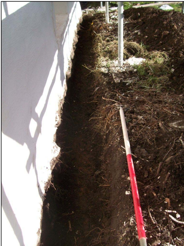
Figure 2b: General shot of trench along northeast half of front elevation from the southwest
