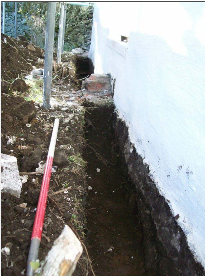
Figure 3b: General shot of trench along southwest half of front elevation from the northeast
