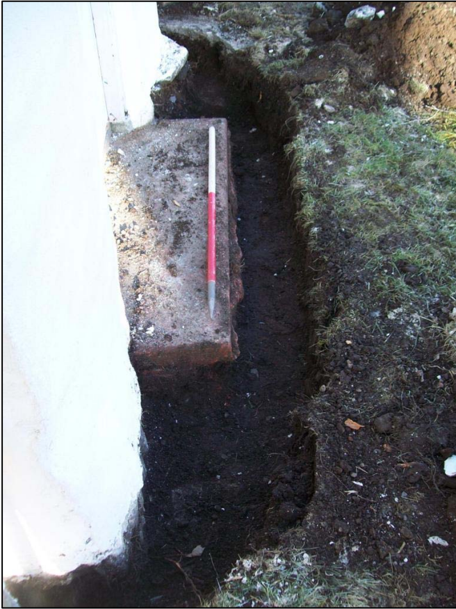
Figure 3a: General shot of trench along front of porch from the southwest
