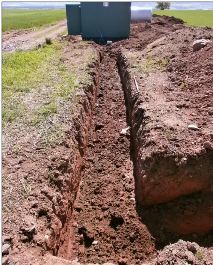
Figure 5b: Trench leading to sub-station and demonstrating (001) and (002) in section (foreground of image).
