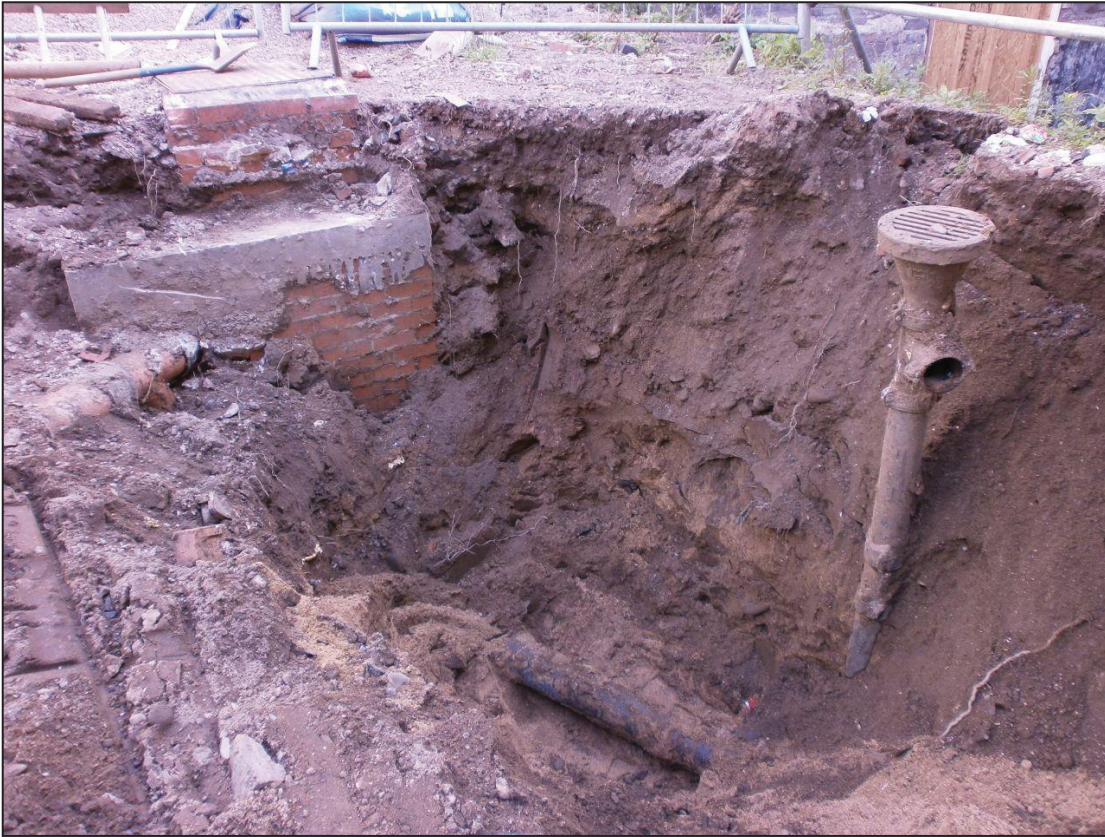
Figure 9a: Demonstrating the highly disturbed deposit (017) and the modern waste water pipe
