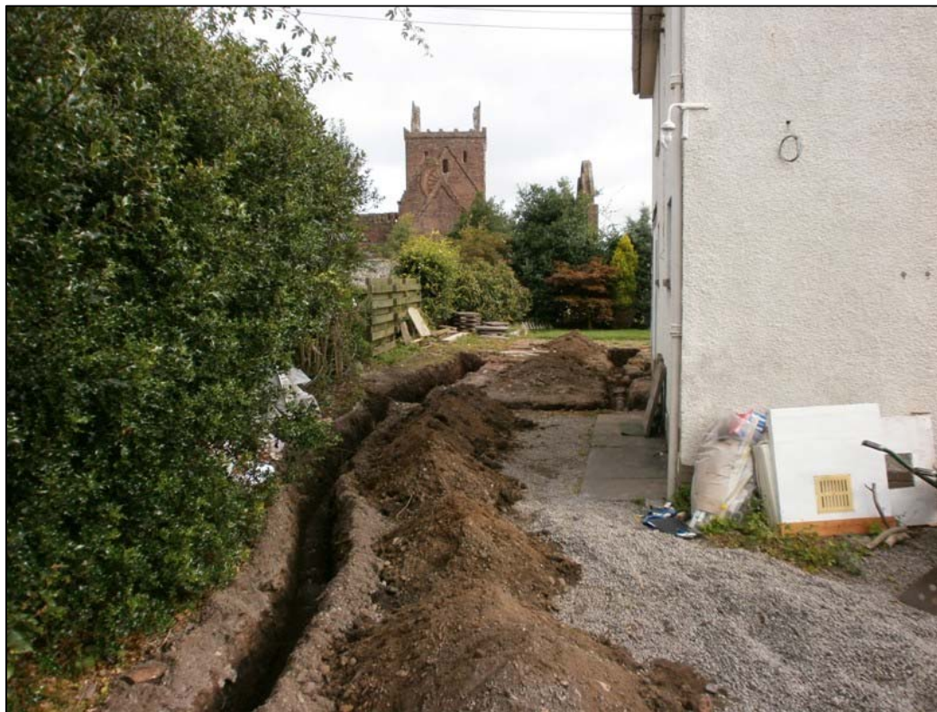
Figure 3a: Oil Line and Water trench running south from outline foundation trench.
