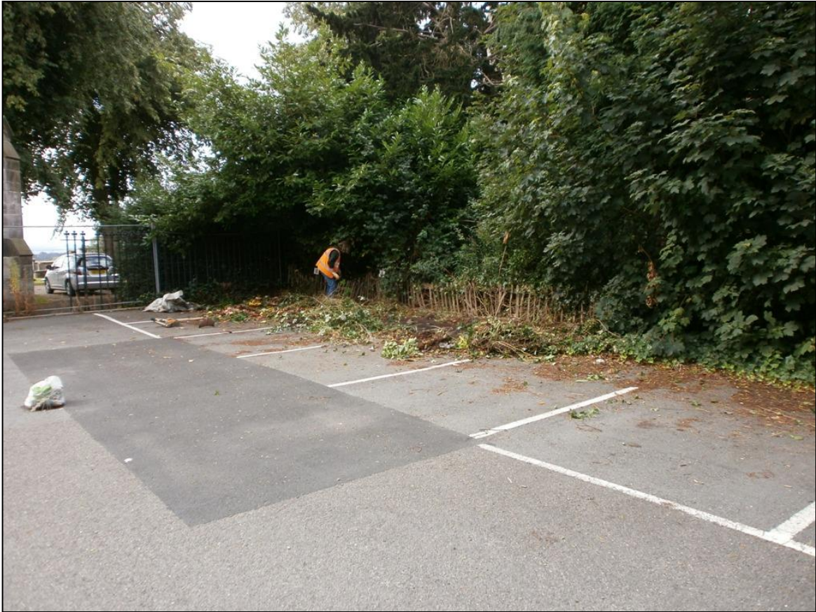
Figure 6a: Site preparation; clearing vegetation along the west edge of the site.
