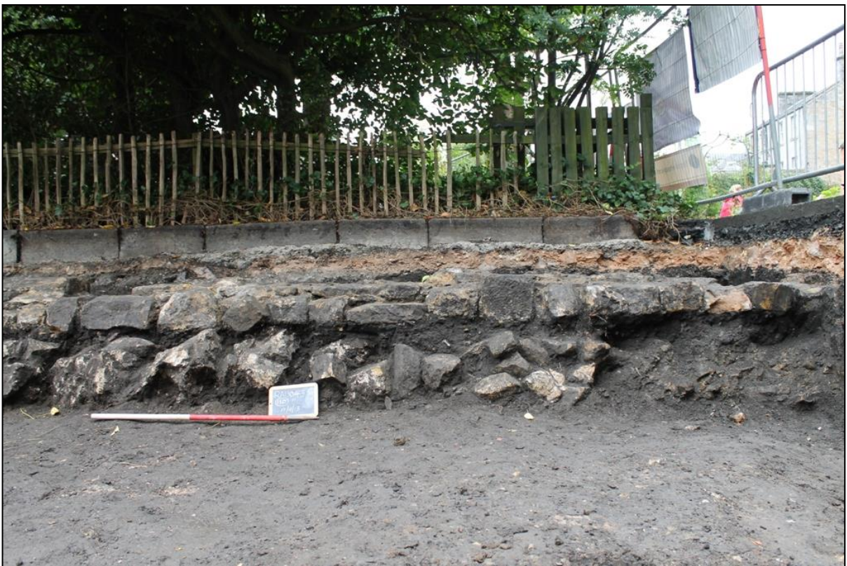
Figure 12b: The east facing section of (110) showing the upper course and foundations.
