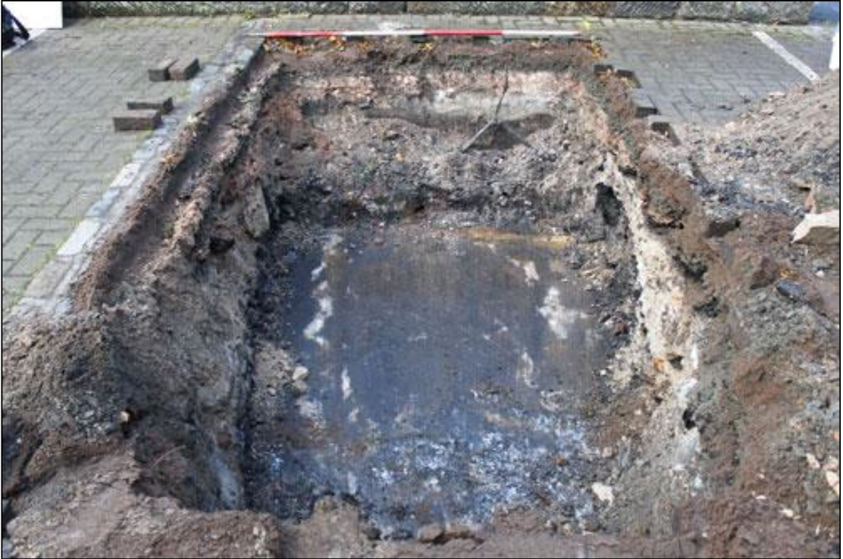
Figure 4a: Trench 4b demonstrating the concrete base and demolition material associated with St Margaret's Hall
