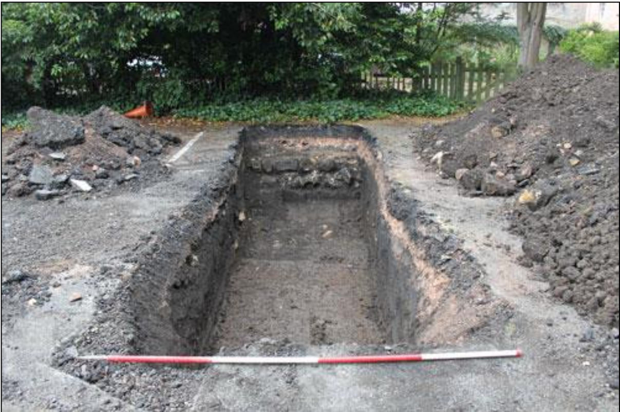
Figure 4b: Trench 1 demonstrating the re-exposed the 19 th century boundary uncovered at the west end of Trench 1
