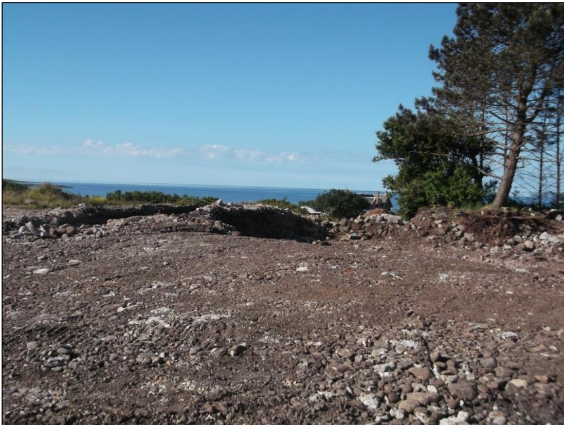
Figure 7: Post excavation view of Trench A within western part of watching brief area. From northeast.
